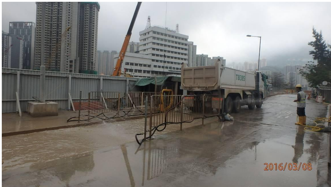
Fig.5 High-pressure water jets were installed at the wheel washing bay
