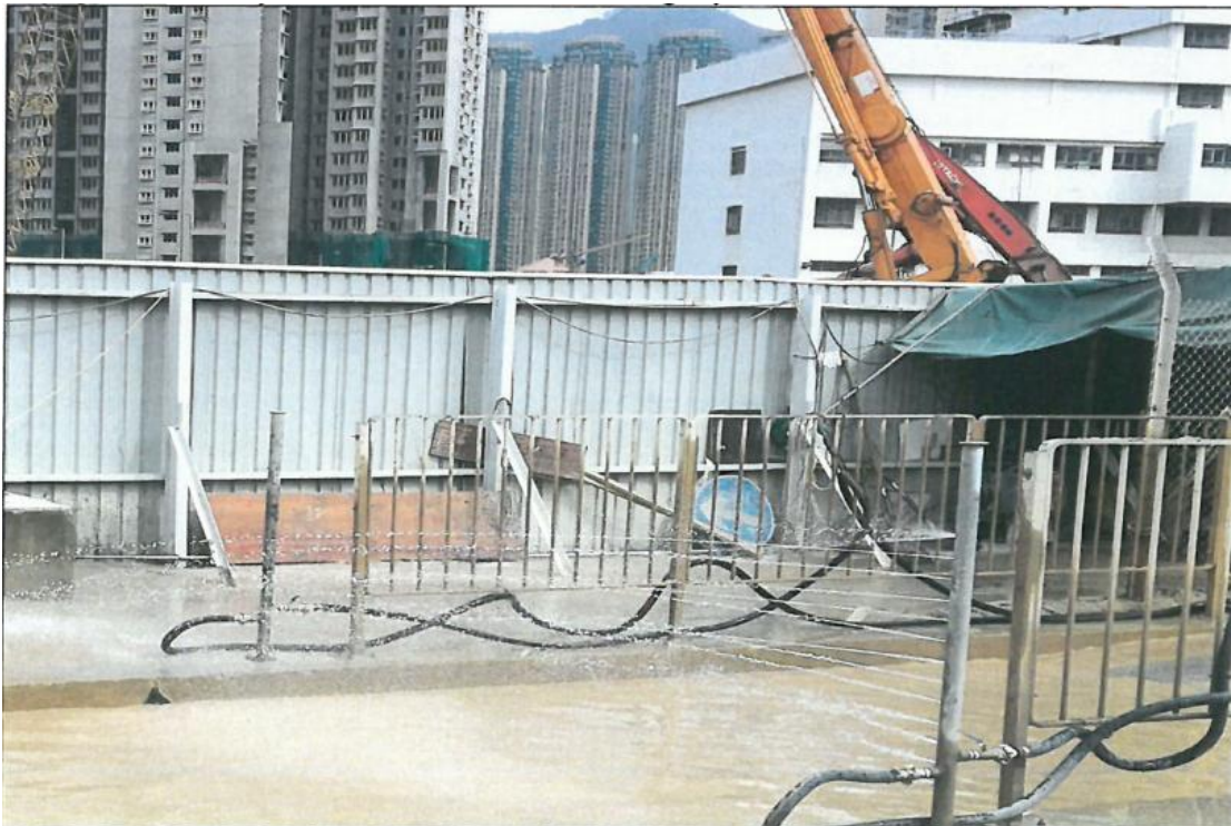
Fig. 4 High-pressure water jets are installed at wheel washing bay. (25 th February 2016)
