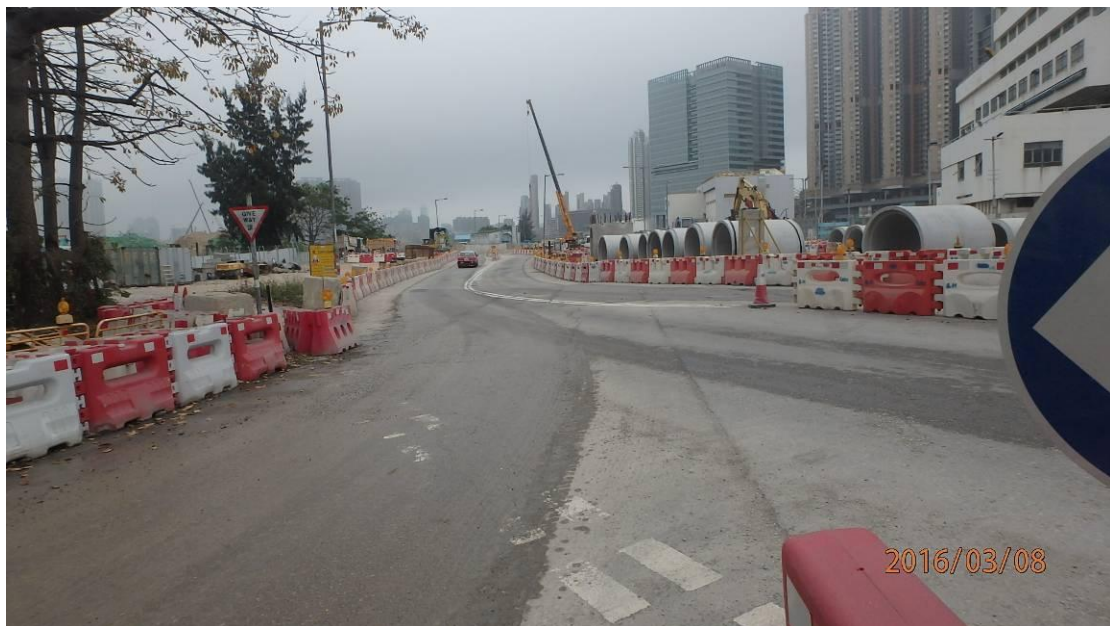
Fig.8 No mud was observed on the haul road near Gate 1 and Concorde Road.
