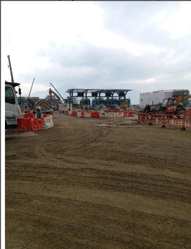
Haul road is wet (Point B)
