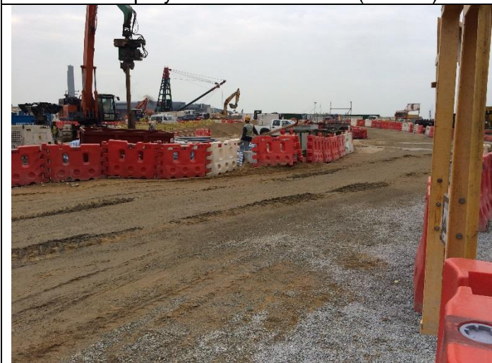
Haul road is wet (Point D)
