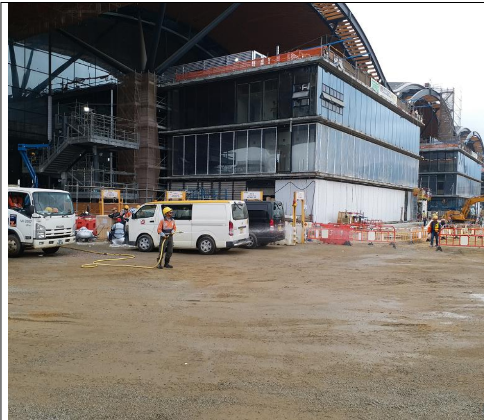
Haul road is wet (Location 1)
