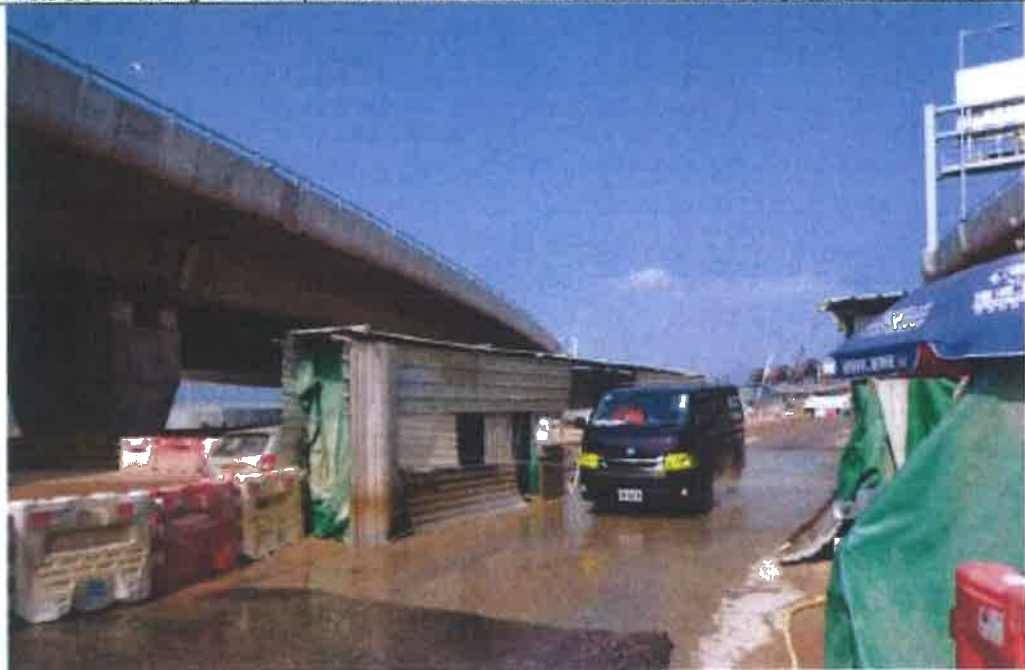
Photo 2.4 – Wheel-washing facilities with high pressure water jet
