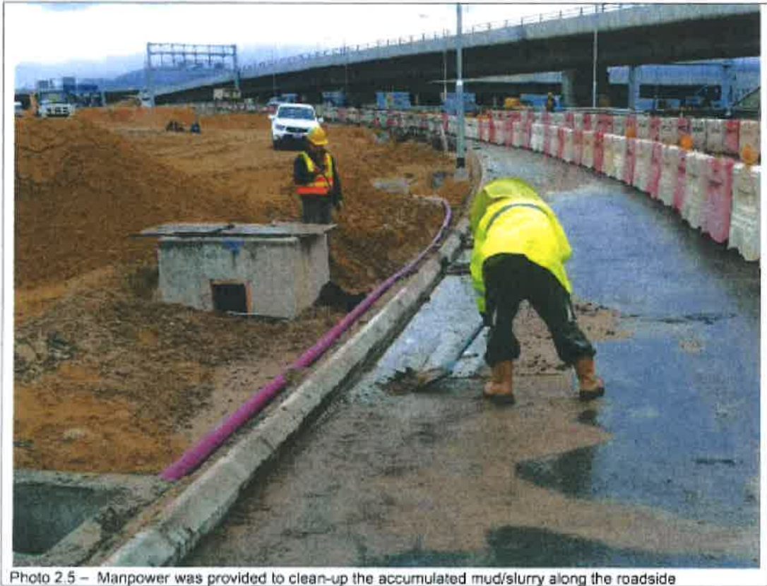
Photo 2.5 – Manpower was provided to clean-up the accumulated mud/slurry along the roadside
