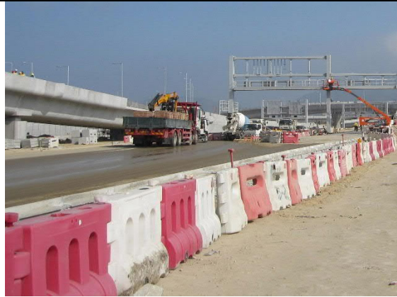
1. Water spray provided for haul roads in the HY/2013/04 site area (near Box Culvert C). No fugitive dust generation was observed.
