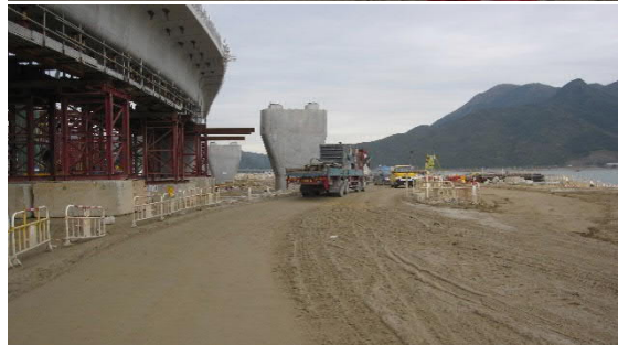
3. Haul roads were wetted in the HY/2013/04 site area (between Box Culvert C and Box Culvert D).
