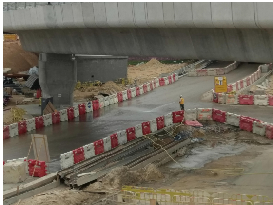
1. Wheel wash facility and water spray provided at HY/2013/04 site boundary for vehicles leaving HY/2013/04 site towards BCF Island site exit.
