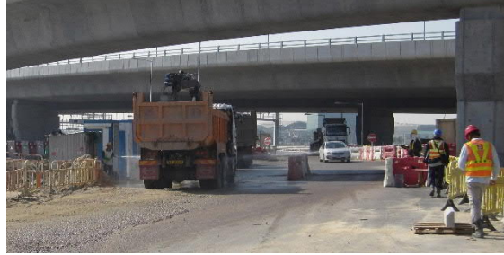
1a. Water spray provided for site vehicles leaving the HY/2013/04 site area towards BCF Island site exit.
