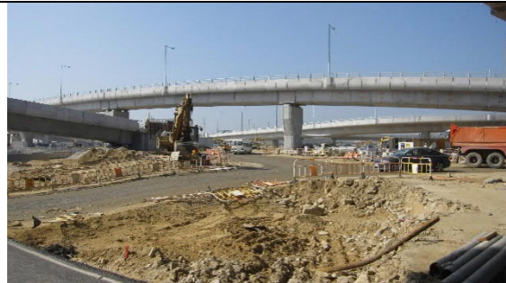
4. Water spray provided for haul roads in the HY/2013/04 site area (near Bridge D9a). No fugitive dust generation was observed.
