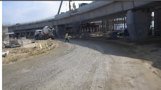
3. Water spray provided for haul roads in the HY/2013/04 site area (near Bridge D10). No fugitive dust generation was observed.
