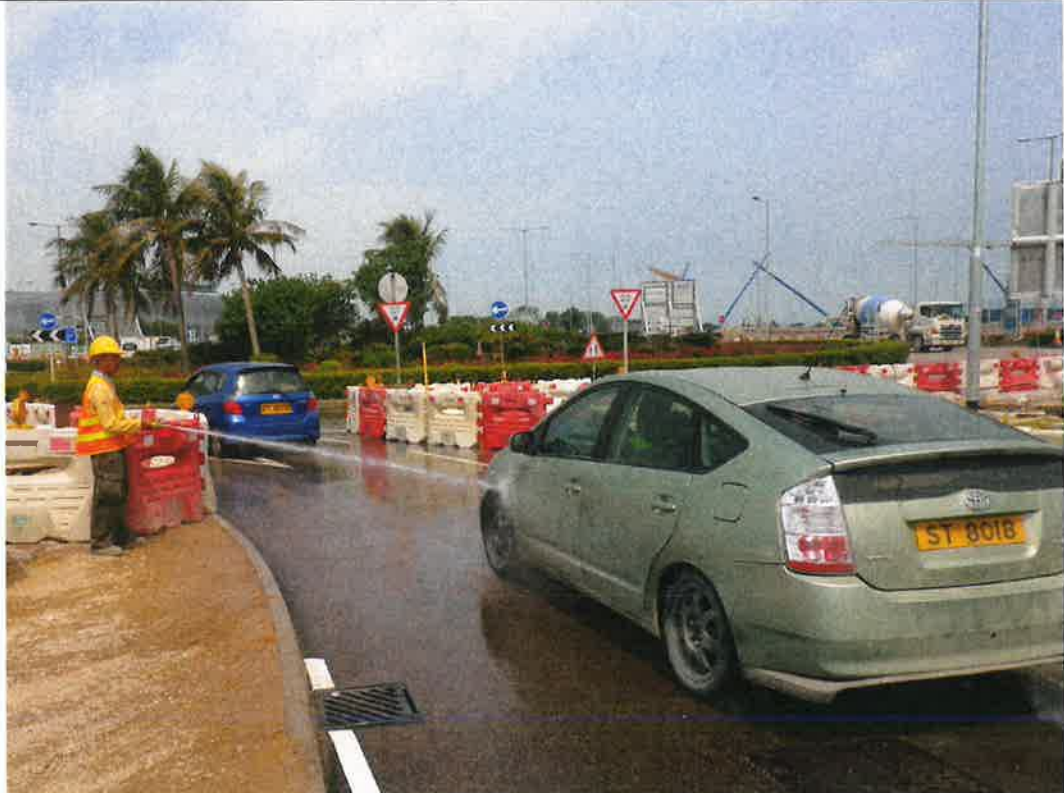
Photo 180315_003 & 004 –Washing facilities with high pressure water jet at the intersection with other contract and the site exit
