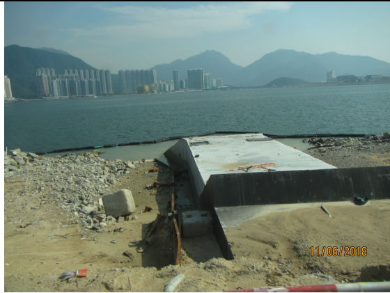
1. Silt curtain at Box Culvert C was observed as secured. No leakage of muddy water into the open waters was observed.
