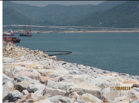
2. Silt curtain at Box Culvert D was observed as secured. No leakage of muddy water into the open waters was observed.
