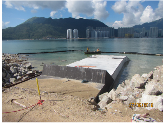
1. Silt curtain at Box Culvert C was observed as secured. No leakage of muddy water into the open waters was observed.
