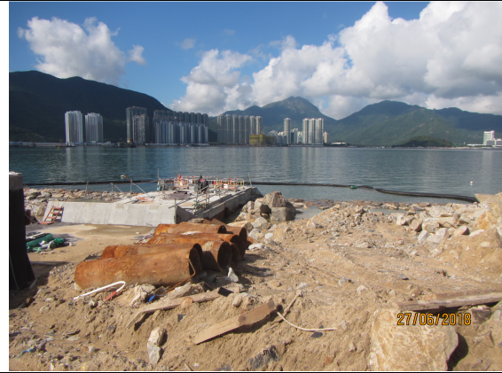
2. Silt curtain at Box Culvert D was observed as secured. No leakage of muddy water into the open waters was observed.
