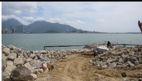
1. Silt curtain at Box Culvert C was observed as secured. No leakage of muddy water into the open waters was observed.
