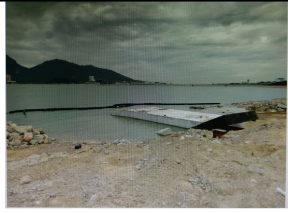
2. 16 June 2018: Silt curtain at Box Culvert C was observed as secured. No leakage of muddy water into the open waters was observed.
