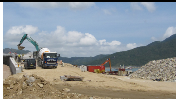
2. Silt curtain at Box Culvert D was observed as secured. No leakage of muddy water into the open waters was observed.
