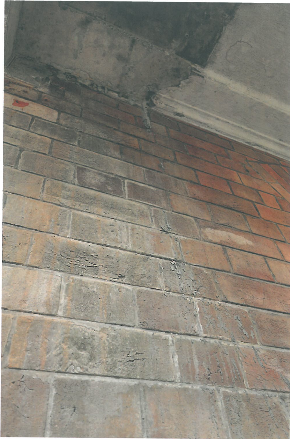
Above, photo taken on 18 th March 2016, showing spilt concrete on the Block 9 Magistracy Terrace (2/F West elevation).
