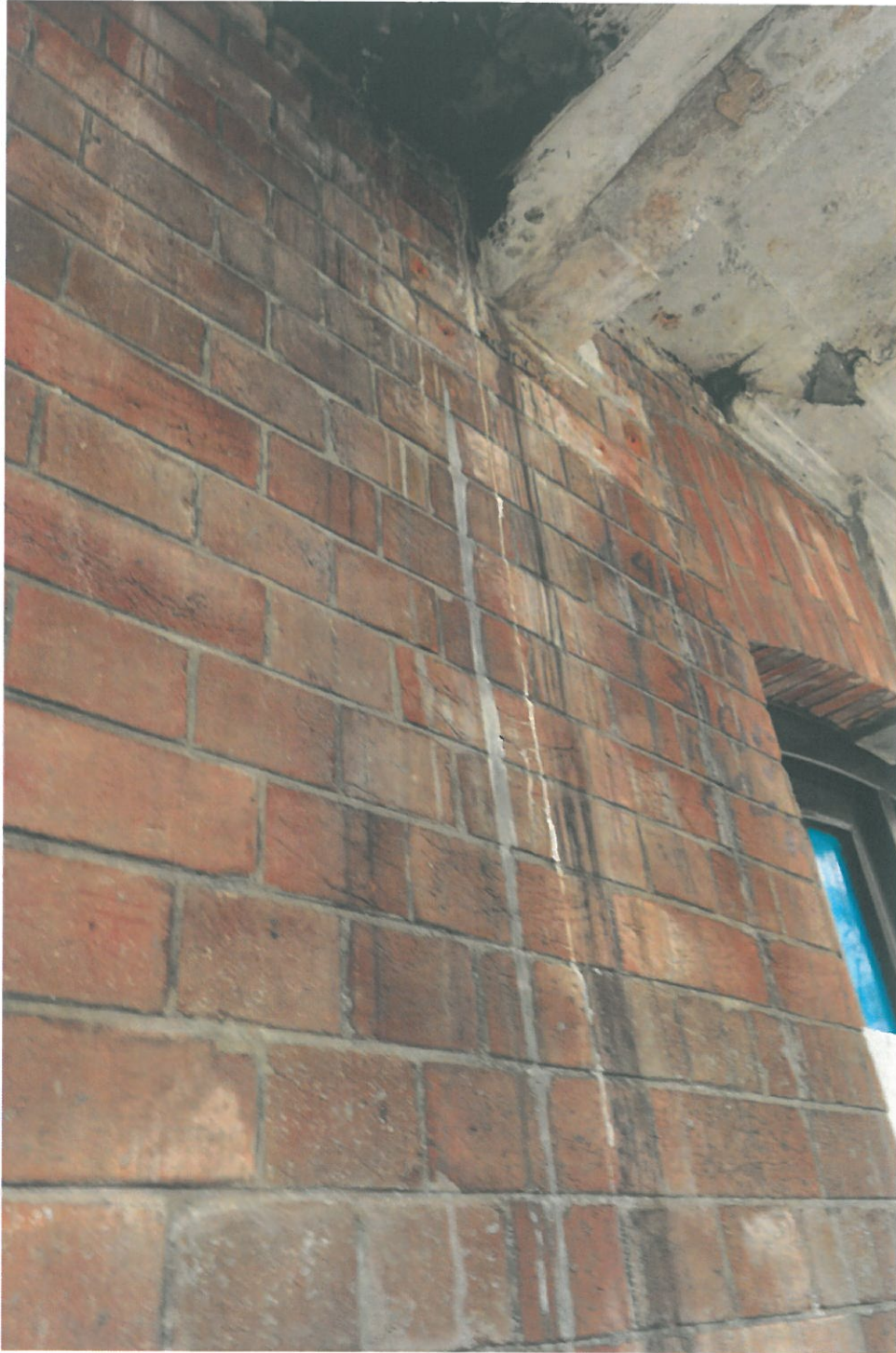
Above, photo taken on 18 th March 2016, showing spilt concrete on the Block 9 Magistracy Terrace (2/F West elevation).
