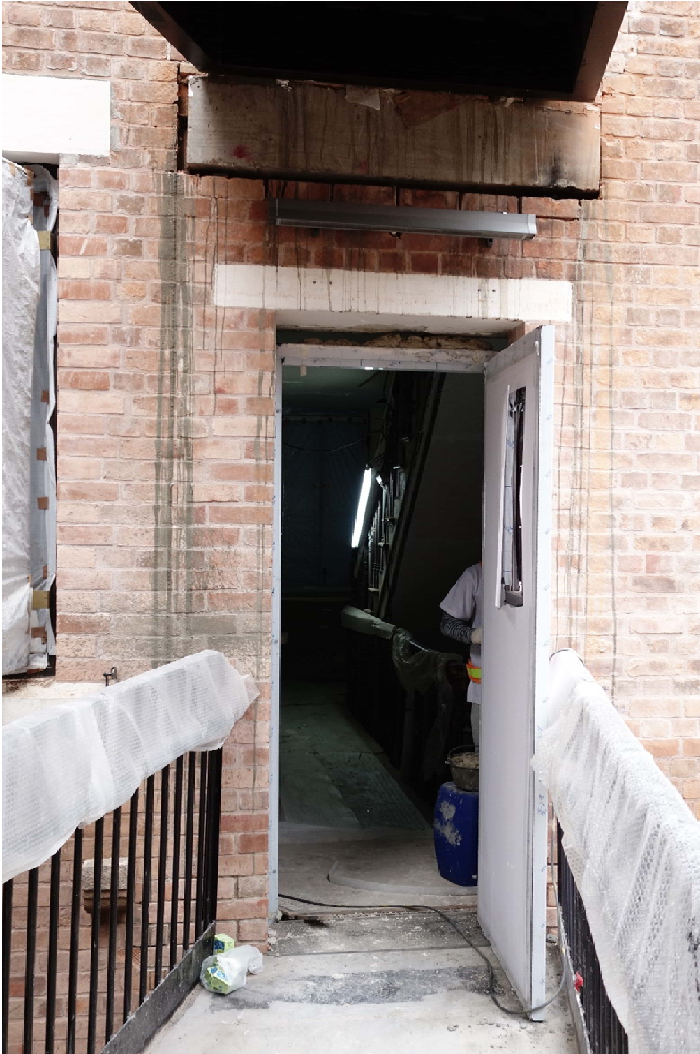
Above, photo taken on 18 th March 2016, showing spilt concrete on the Block 7 North elevation (1/F).
