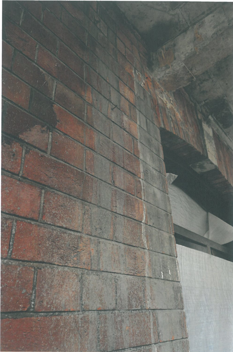
Above, photo taken on 18 th March 2016, showing spilt concrete on the Block 9 Magistracy Terrace (2/F West elevation).
