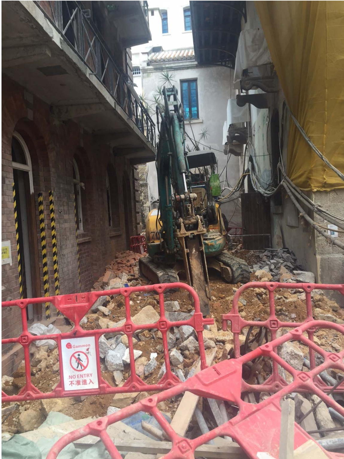
Above, photo taken on 5 th November 2015, showing site works on the Magistracy Terrace (West). No protection was provided to the granite steps nor the masonry walls.
