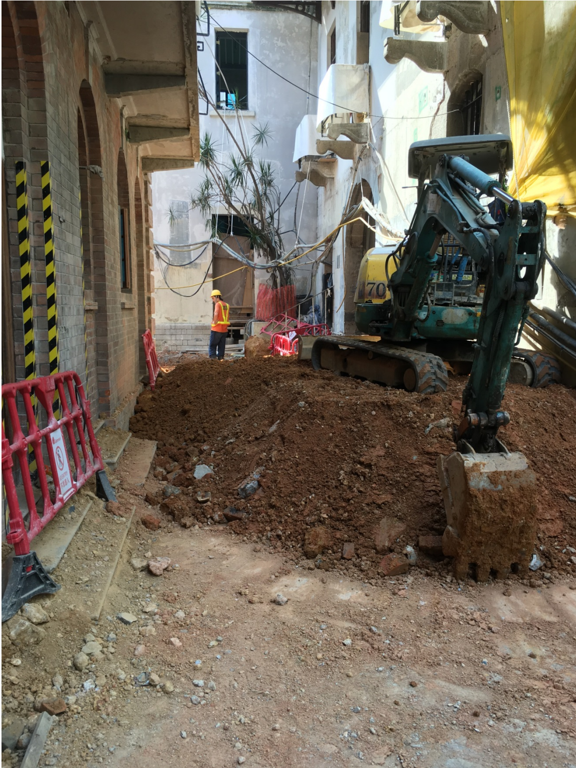
Above, photo taken on 23 rd November 2015, no improvement had been made to protect the surrounded building fabric.
