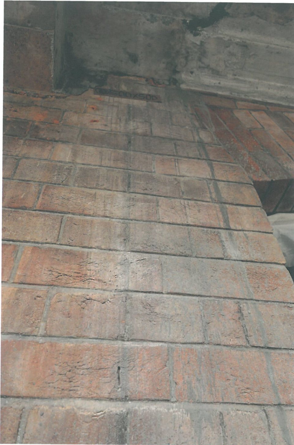
Above, photo taken on 18 th March 2016, showing spilt concrete on the Block 9 Magistracy Terrace (2/F West elevation).
