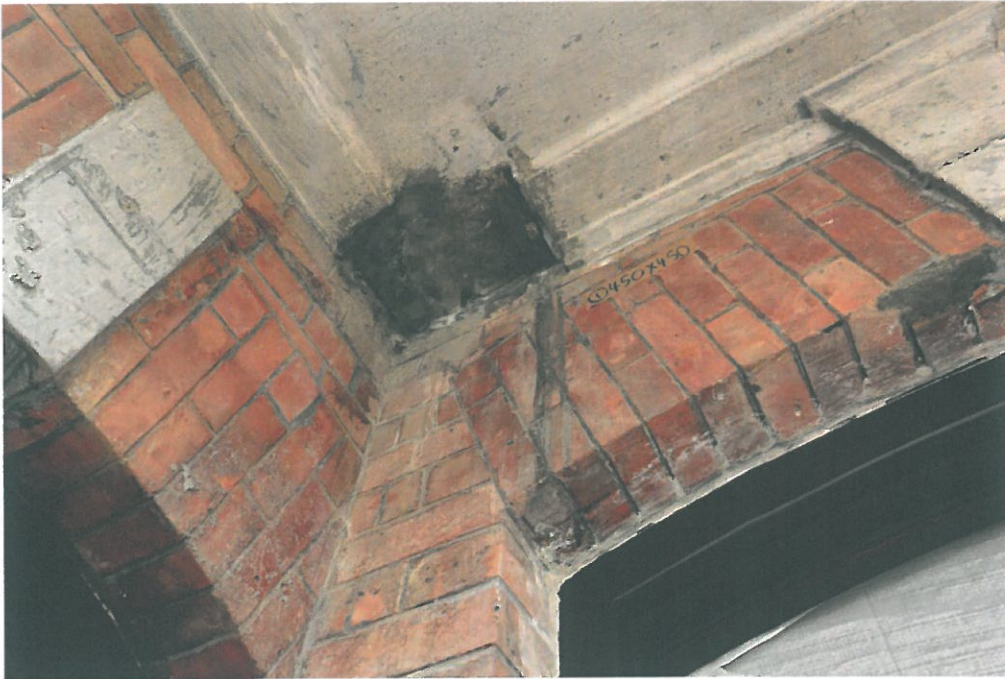
Above, photo taken on 18 th March 2016, showing spilt concrete on the Block 9 Magistracy Terrace (2/F West elevation).
