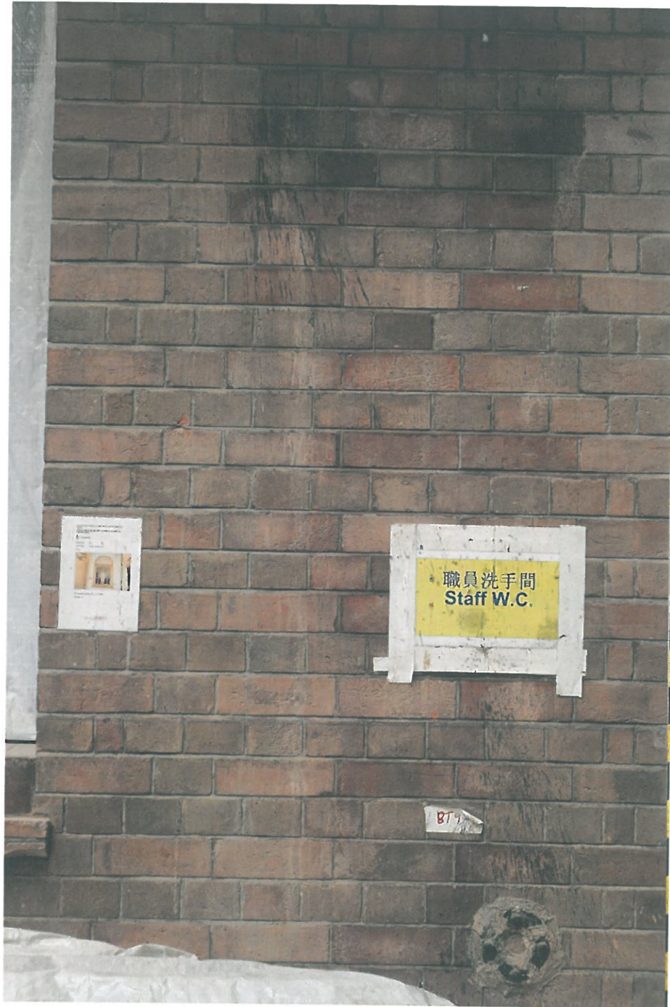
Above, photo taken on 18 th March 2016, showing spilt concrete on the Block 9 Magistracy West elevation (G/F).
