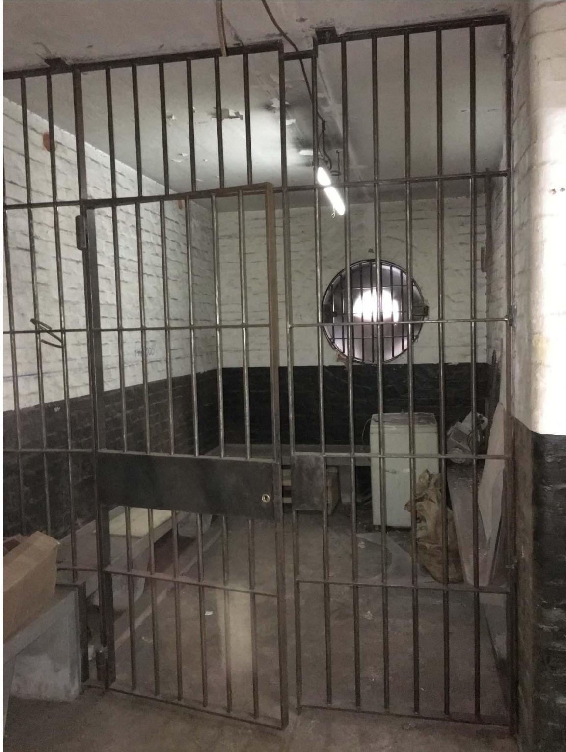
Above, photograph taken on 25 th February 2016, the conduits, lighting, mesh and fan on the window, paint on the metal gate were incorrectly removed. Removal of mesh had damaged adjacent brickwork.
