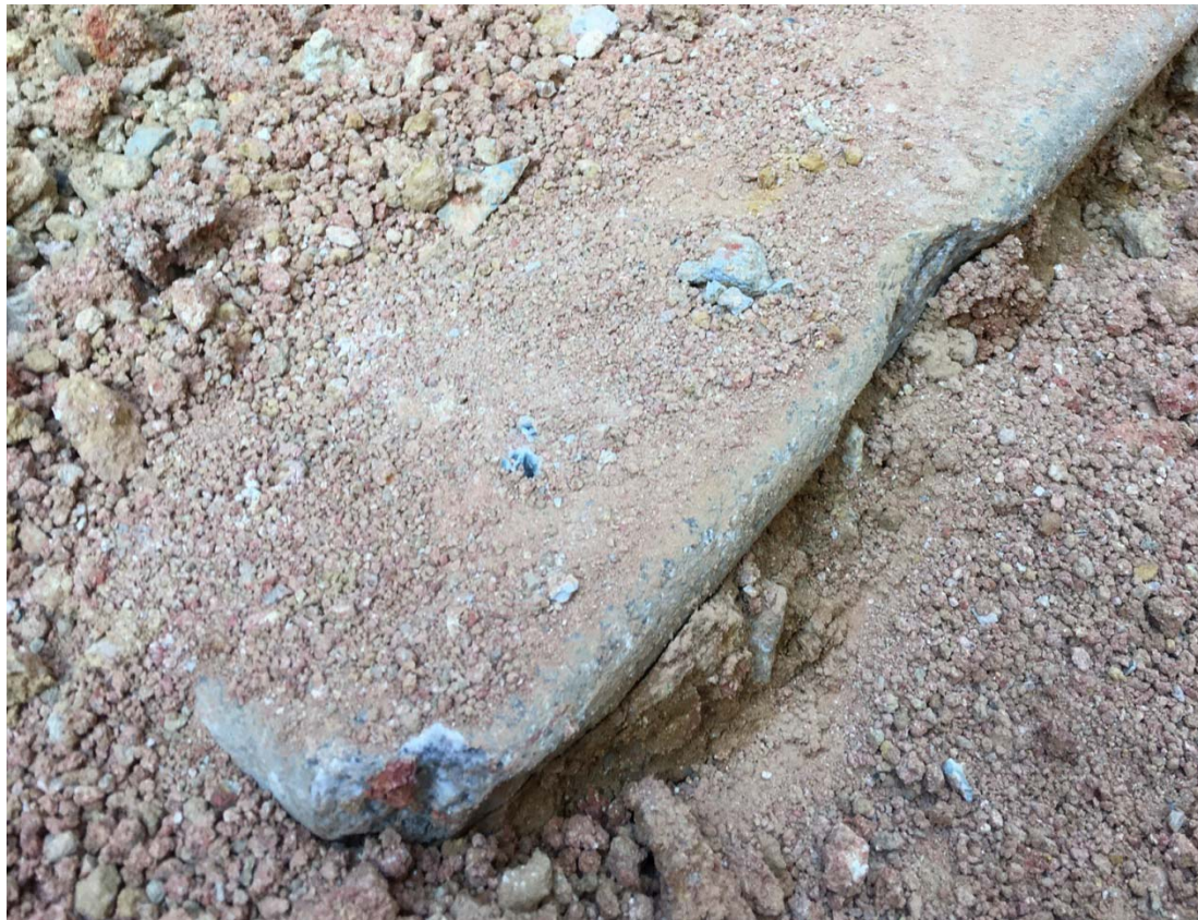
Above, photo taken on 23 rd November 2015, showing granite steps at 09/WG/04 damaged by site works.
