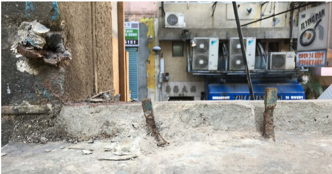
Above, photograph taken on 25 th January 2016, showing the balusters of the fence was cut.
