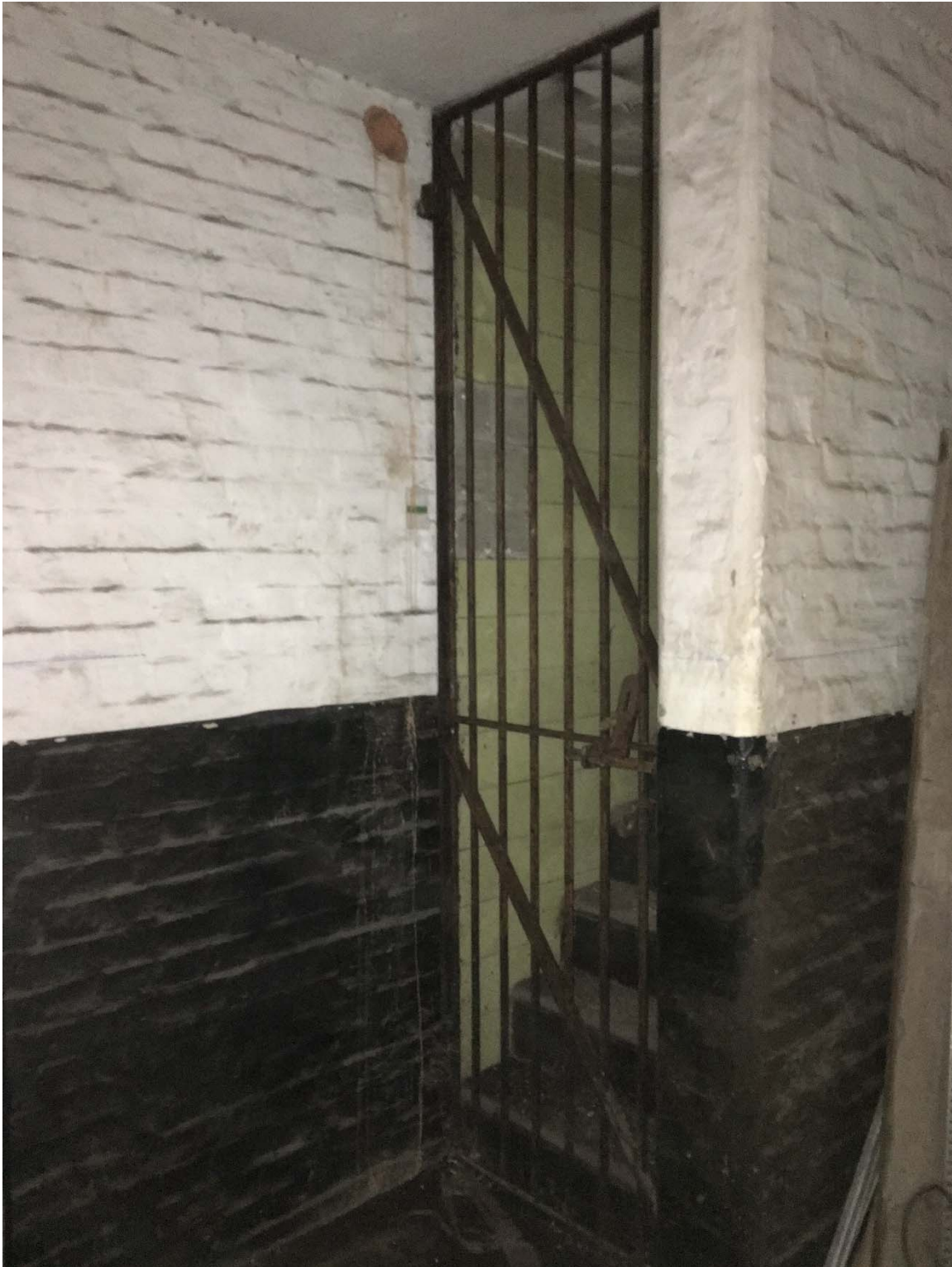
Above, photograph taken on 25 th February 2016, the mesh and the paint were incorrectly removed from the gate.
