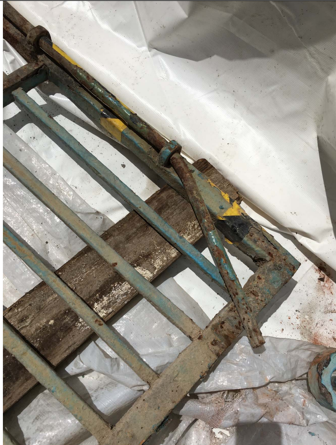
Above, photo taken on 21 st July 2016, showing the drop bolt on the right hand side leaf was bent.
