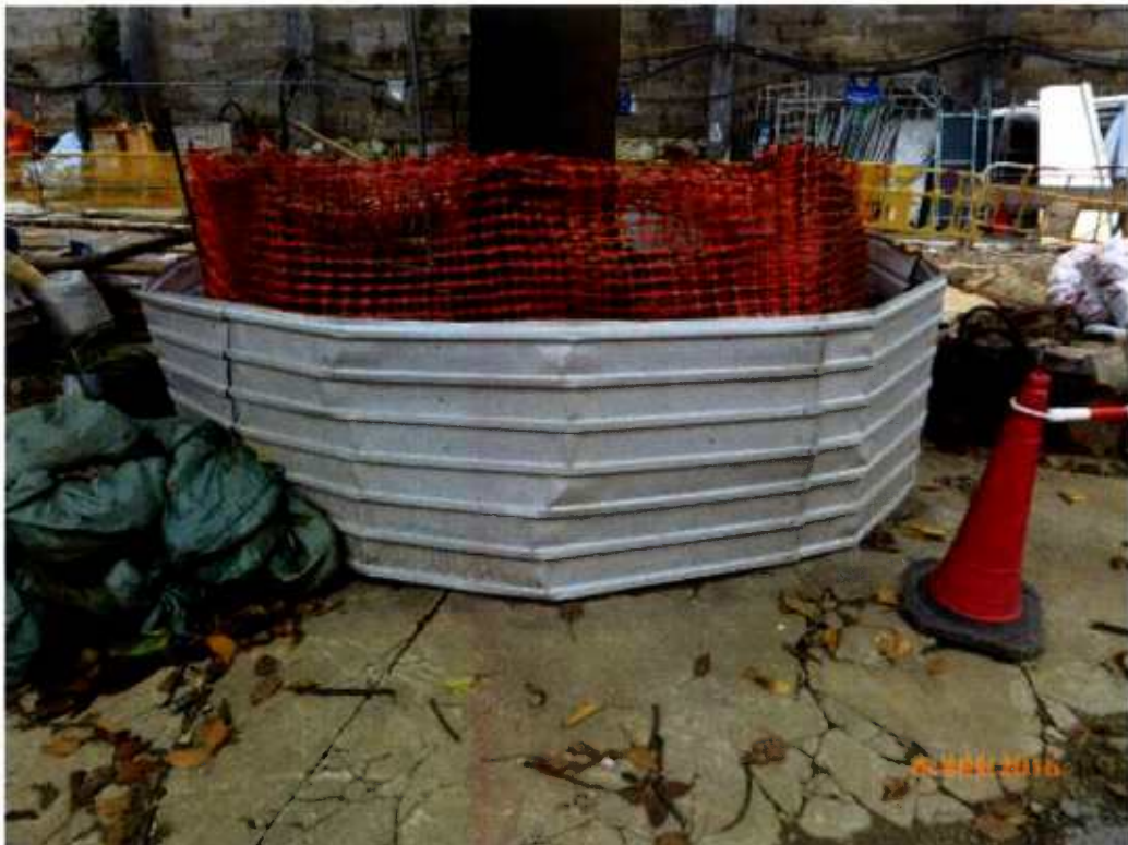
Fig. 9 The small cordon zone is in good order at the time of inspection.
