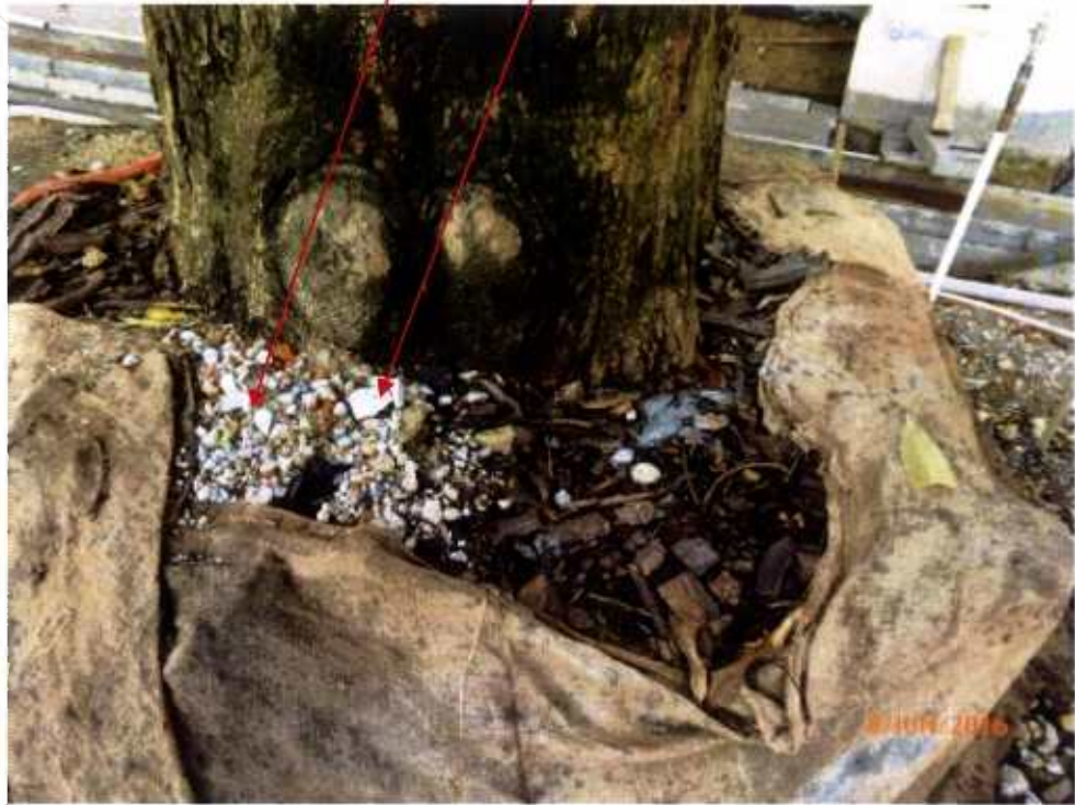
Fig 2. Root collar is normal. The bare roots have been covered with Hessian Clothes. Lots of construction debris are found at the planter.
