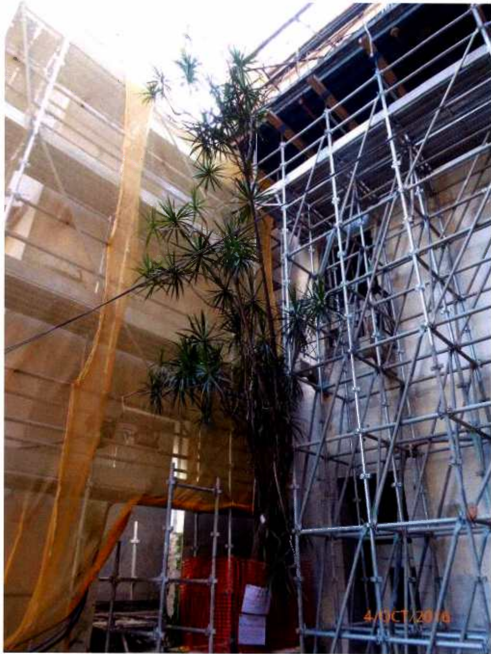
Fig. 12 Overall view of Tree-11 during inspection on 4 th October 2016.
