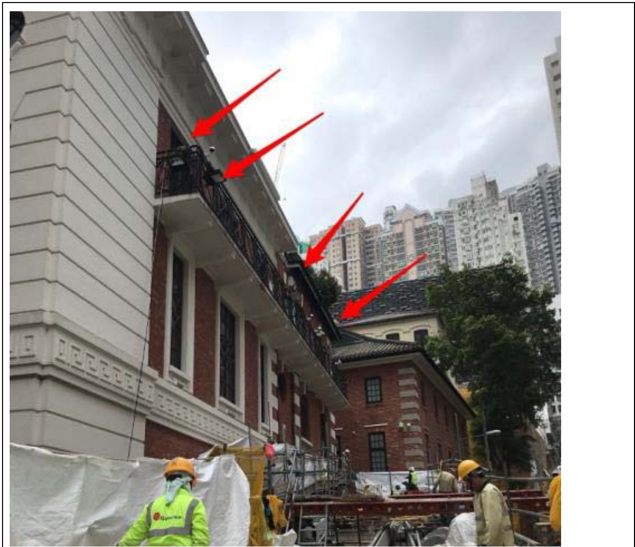
Photo 1: Four Light fittings on the external façade of Block 1 facing Old Bailey Street
