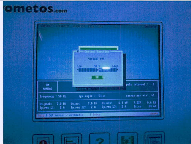
Typical manual mode setting for 50% ignition angle and check voltage and current of ESP Ioniser unit on screen after 30 minutes.
