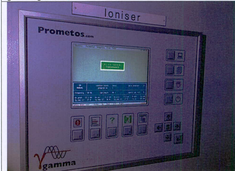
Typical manual mode setting for 40% ignition angle and check voltage and current of ESP Ioniser unit on screen after 30 minutes.
