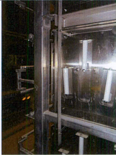
End view on typical common earth tape connected with ESP modules on rack at APS plant room in B2 of EVB
