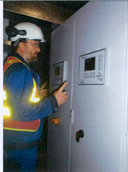
View on energizing of HV control panel (Ionizer) in auxiliary plant room in B2 of EVB
