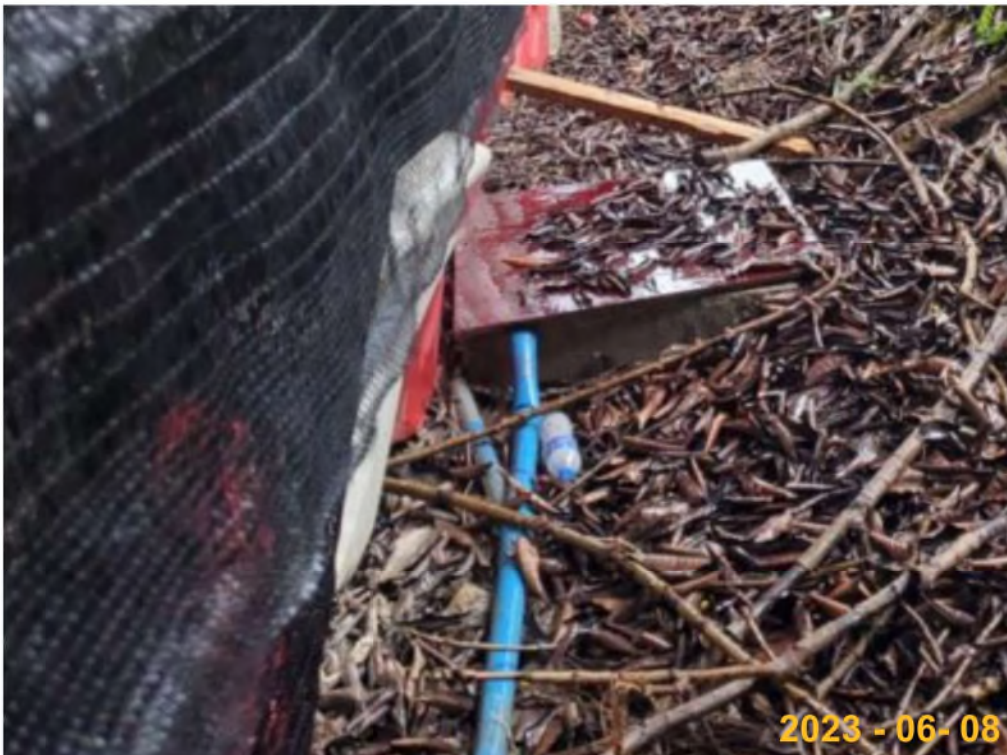
At Zone 3, a blue pipe was found and connected with the drainage system, no treatment facility was found near by the pump and blue pipe.
