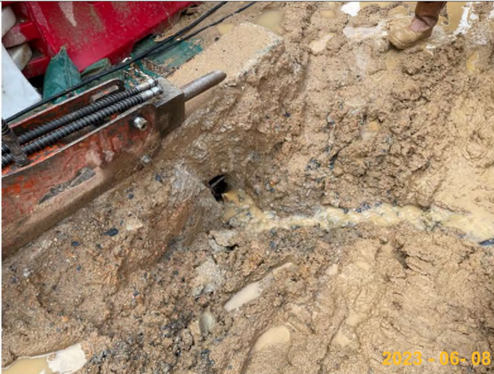
At Zone 4, N4, untreated muddy water surface run-off was observed, the water directly discharges into a guile without any treatment.
