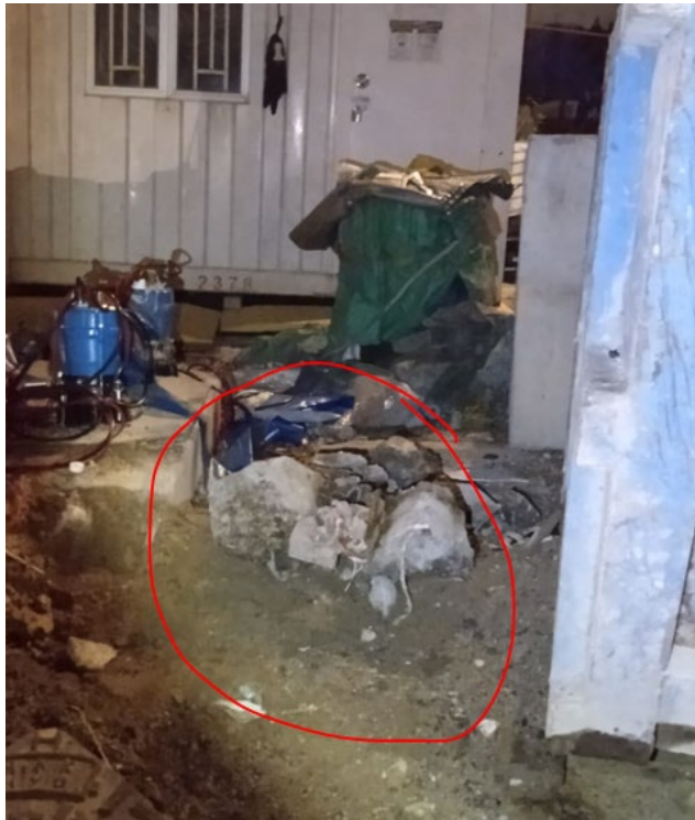
Photo 3 – CCZJV removed rubbish and debris from the blocked manhole (photo date: 20^21 June 2023)
