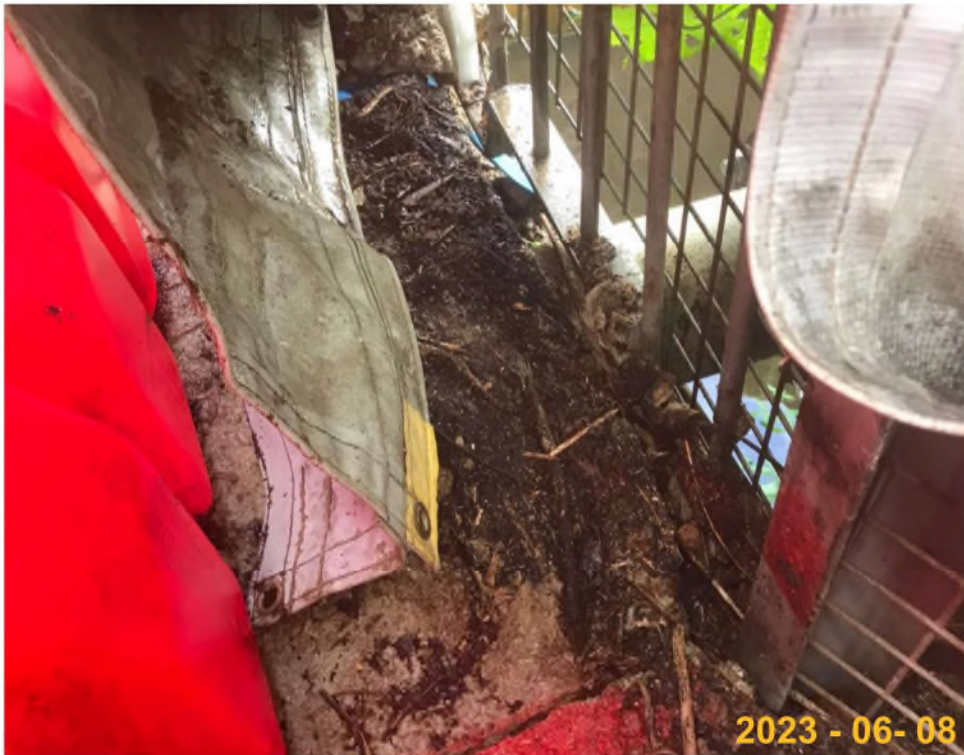
At Zone 4, N4, untreated muddy water discharge was found through the blue pipe to the MTR area, no treatment facility was found near by the pump and blue pipe.
