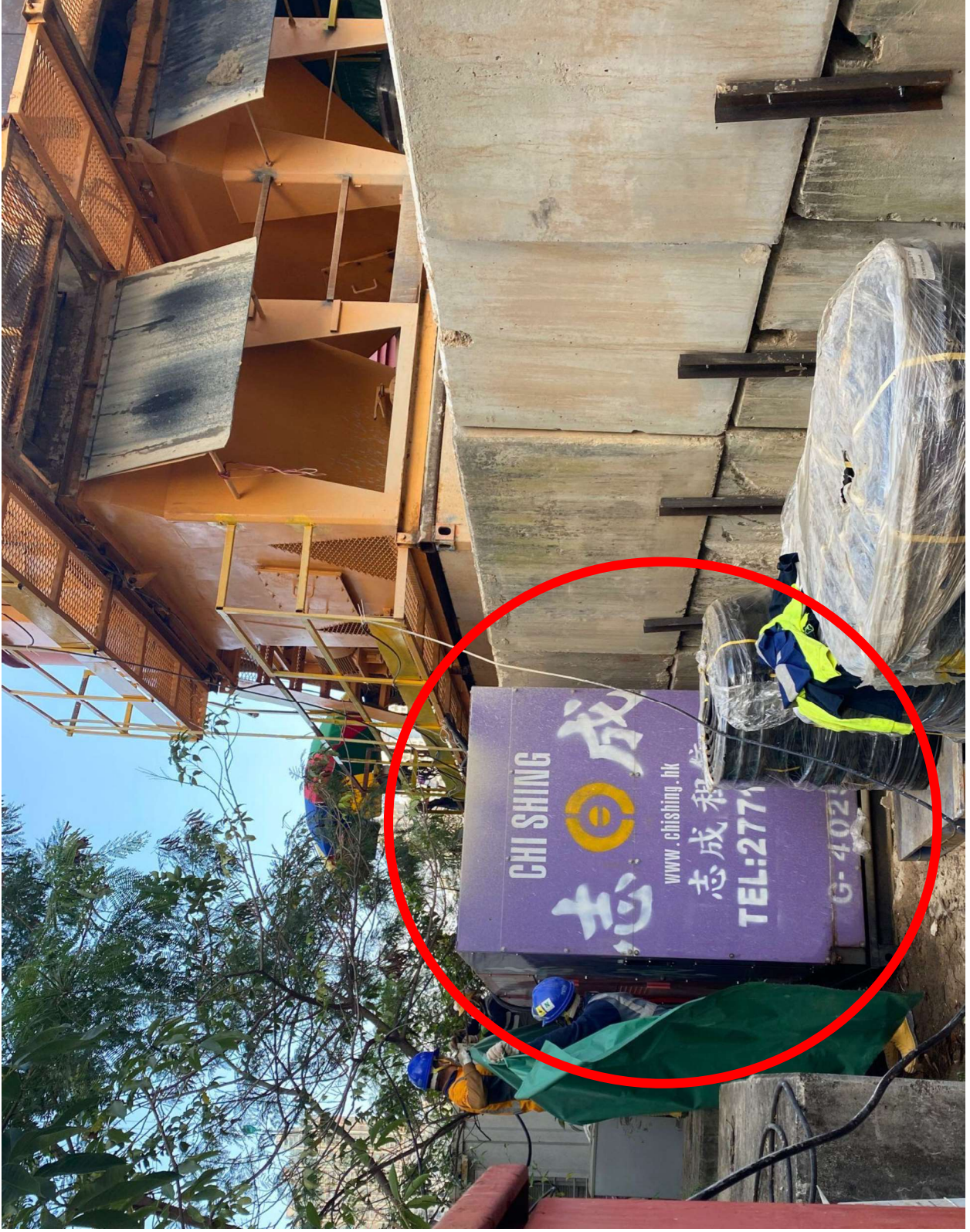
Remark 2: Noise source: generator
