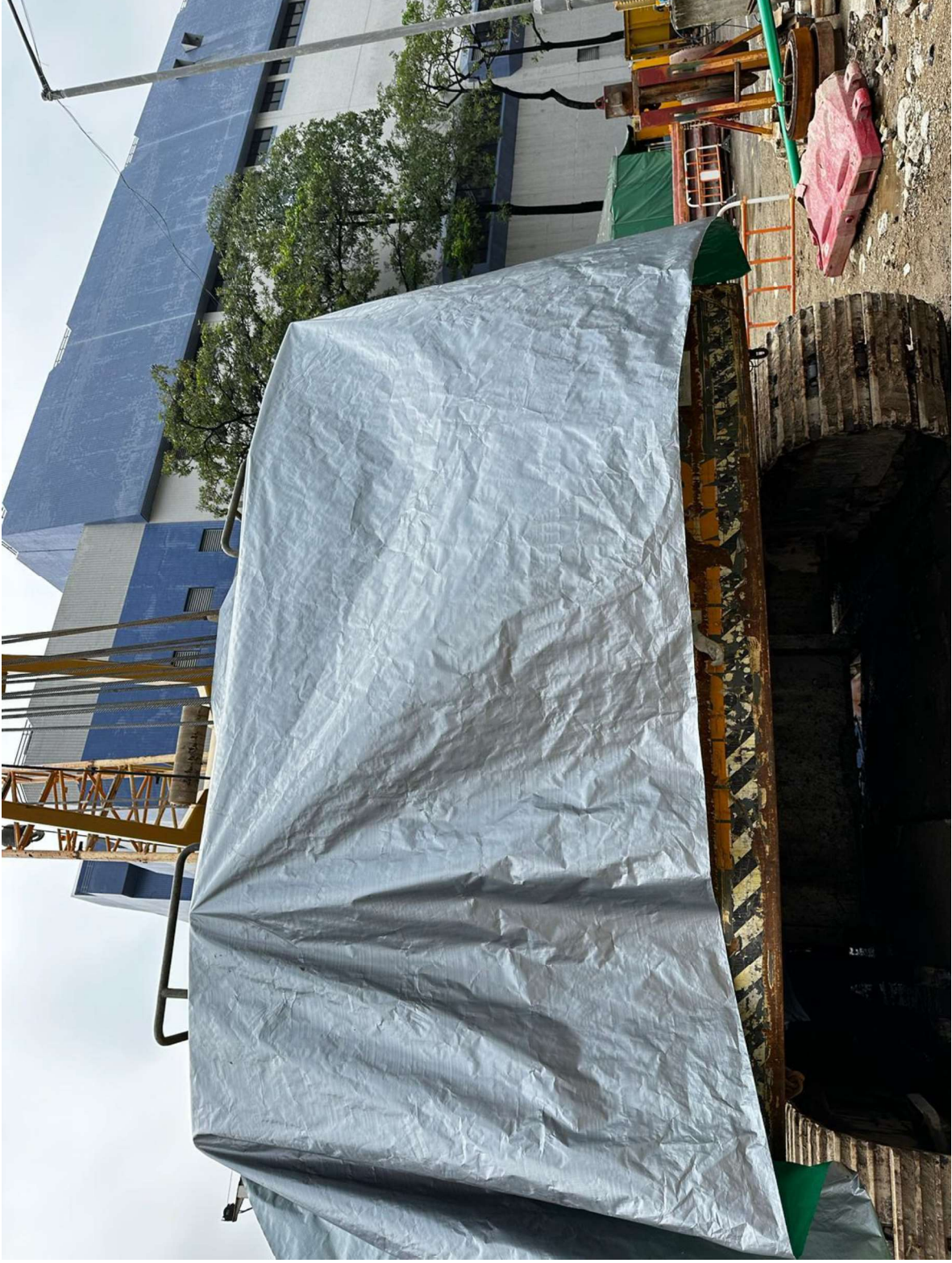
Remark 3: Additional noise canvas at the engineering part of the mobile crane
