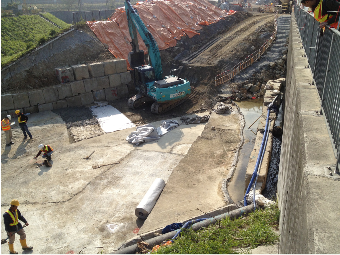
Water leakage has been remedied. No more river water enters the construction site. (Date: 23 December 2013)
