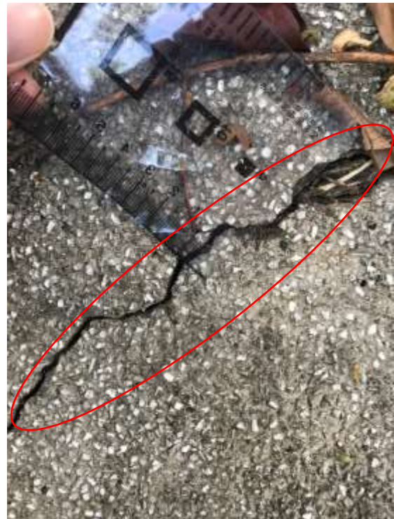
2A-D1(2) - Wide Crack on Surface (Length:1000mm/Width:2.5mm)
