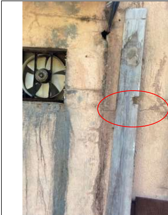
5A5-D8(2) – Moderate Crack on Wall Surface (Length:400mm/Width:1.80mm)
