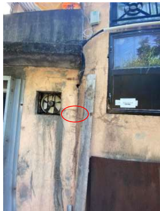
5A5-D8(1) – Moderate Crack on Wall Surface (General View)
