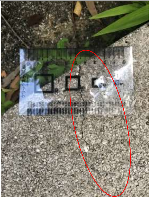
2A-D3(2) - Fine Crack on Surface (Length:200mm/Width:0.65mm)
