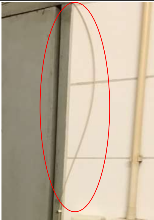
5A5-D9(2) – Moderate Crack on Wall Surface (Length:300mm/Width:1.80mm)
