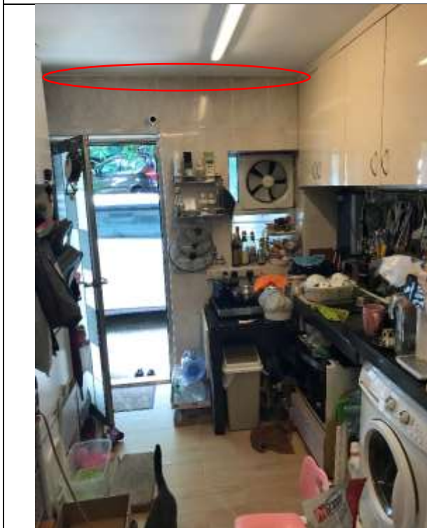
5A2-D2(1) – Spalling between Wall & Ceiling
