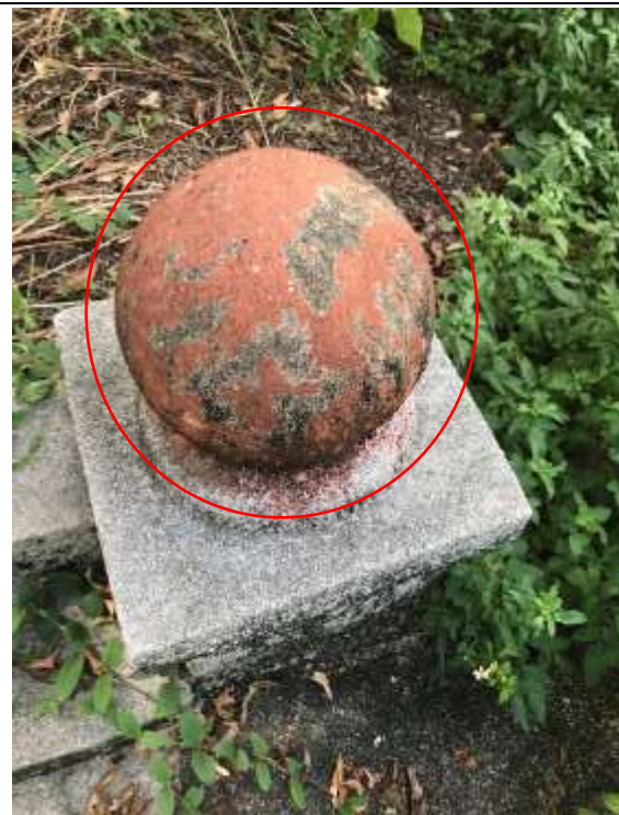
2A-D2(2) – Peeling Paint from Surface
