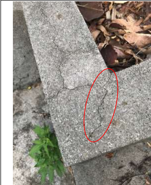
2A-D4(1) - Fine Crack on Surface (General View)
