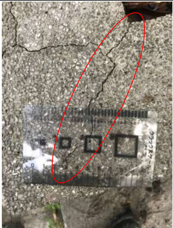
2A-D4(2) - Fine Crack on Surface (Length:200mm/Width:0.80mm)
