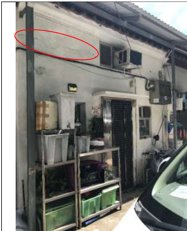
5A2-D1(1) - Crack on Surface
