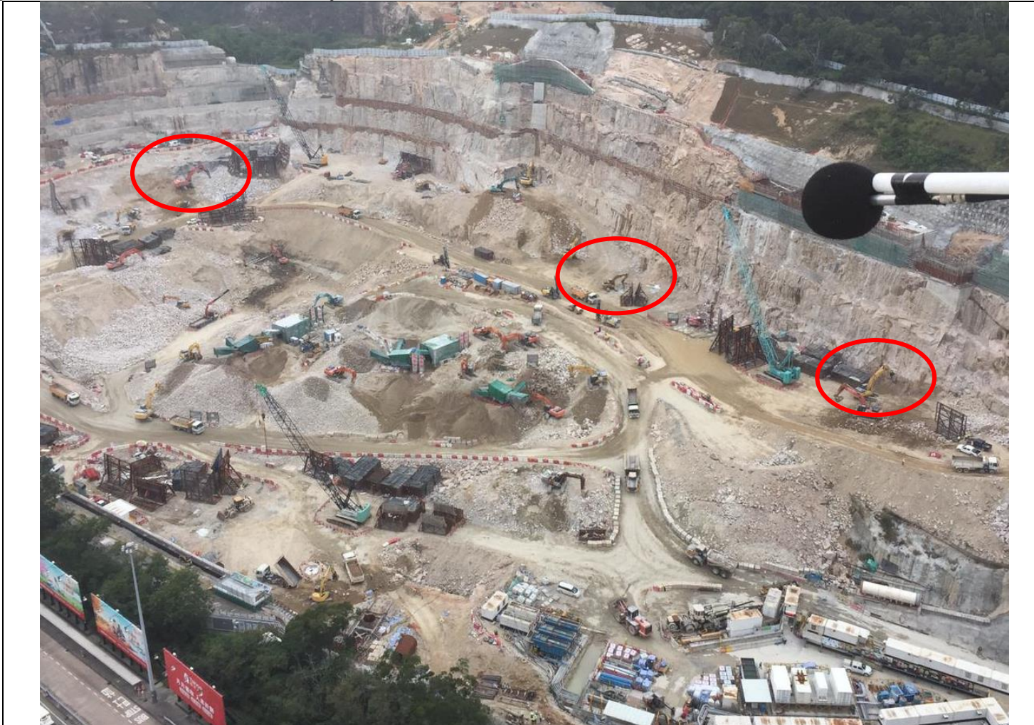
Photo 1 Breaker operation in Portion II
