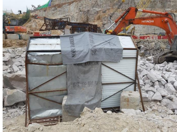
Photo 9, Photo 10 and Photo 11 Movable noise barrier (3m by 3m with 1m cantilever at a tilting angle of 45 degrees) implemented on-site for Portion II
