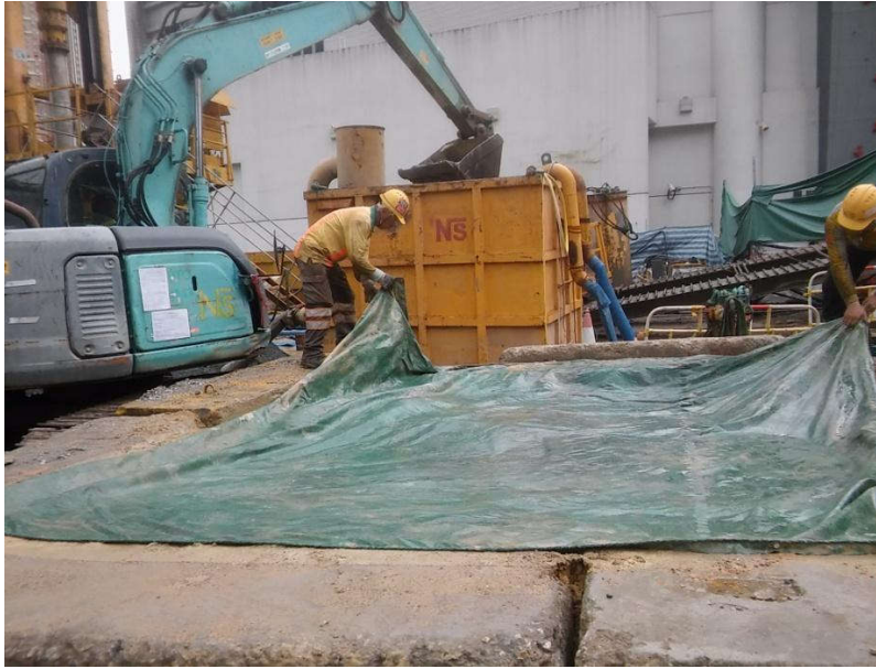
Stockpile Should be proper cover with tarpaulin.
