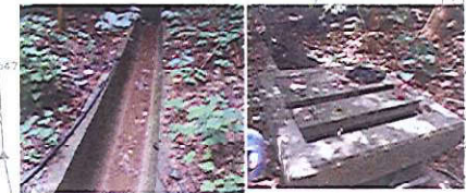
Manhole Inspection for Silt measurement, we have regular cleaning the channel weekly or in an emergency
