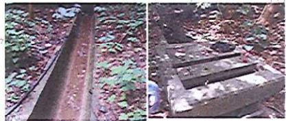
Manhole Inspection for Silt measurement, we have regular cleaning the channel weekly or in an emergency
