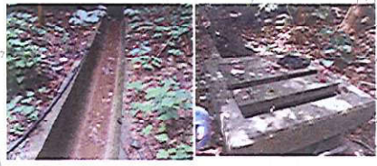
Manhole Inspection for Silt measurement, we have regular cleaning the channel weekly or in an emergency
