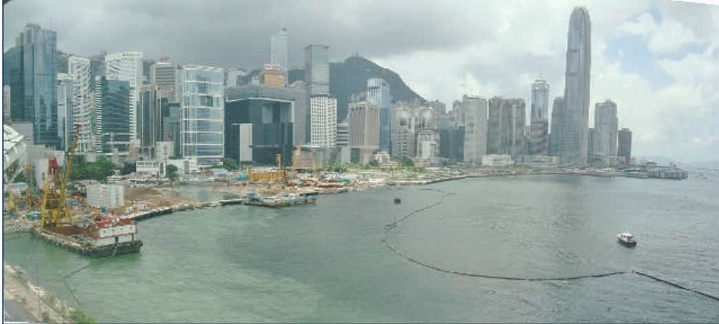
Central – Wan Chai Bypass - seawall separation using heavy non-woven geotextile Bontec SNW120
