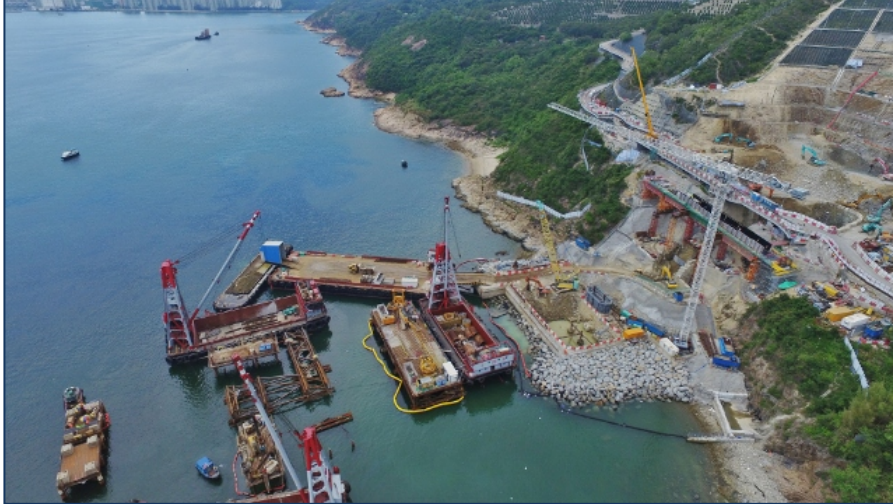
TKO - Lam Tin Tunnel - Main tunnel and associated works using DSP silt curtain
