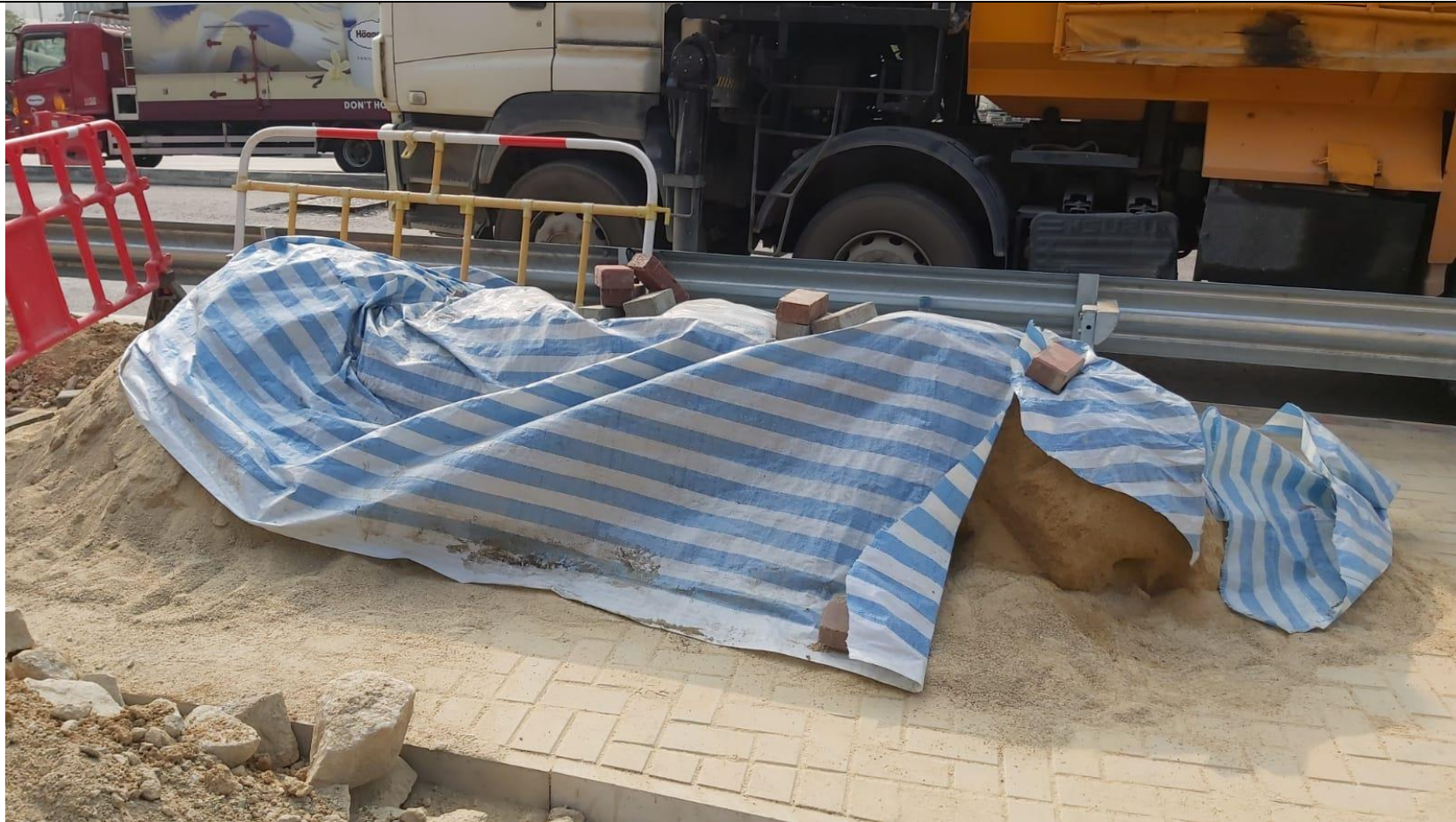
Photo 4 – Mitigation measures implemented on footpath near the roundabout of TKO-LTT (Taken on 18 Mar 2023)
