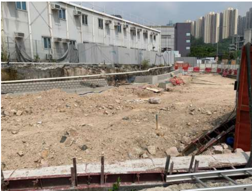
Photo 7 & 8 – Observation of air-quality-related environmental deficiency made by Environmental Team and Independent Environmental Checking on 29 Sep 2021. Stockpile of dusty material shall be covered at WCA (upper) and regular watering shall be applied at Cha Kwo Ling Road (lower).
