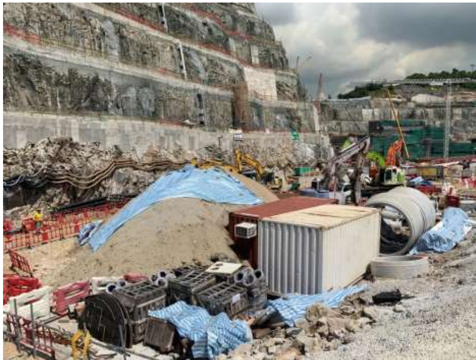
Photo 5 & 6 – Observation of air-quality-related environmental deficiency made by Environmental Team on 15 Sep 2021. Dusty material was leaking from the fabric attached to the tail of rock drill and a trail of dust was left behind (upper) stockpile of dusty material without fully covered (lower).
