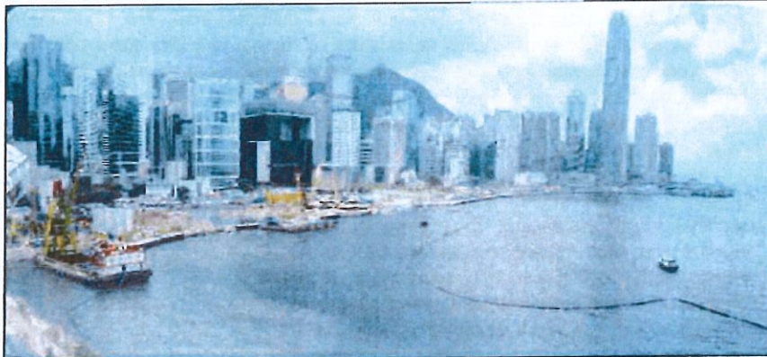
Central – Wan Chai Bypass - seawall separation using heavy non-woven geotextile Bontec SNW120
