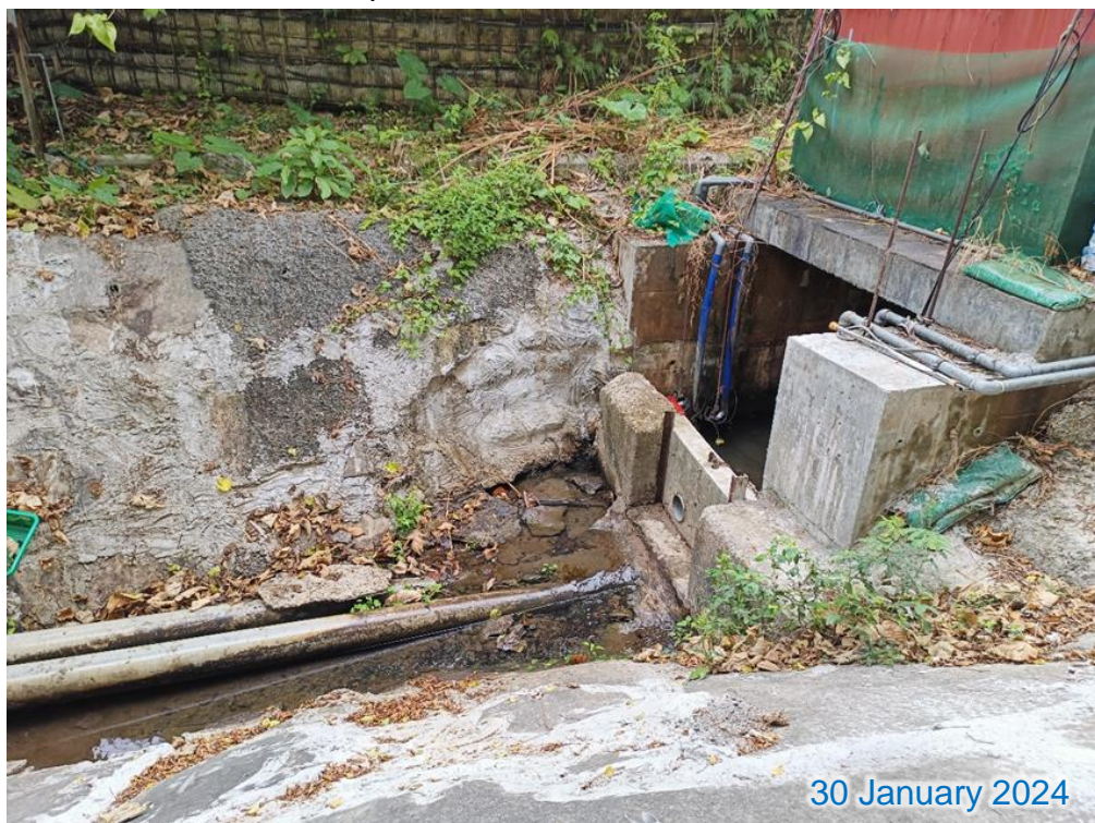
Photo 1 Installation of barrier at the drainage channel to intercept site runoff and pump the wastewater to the sedimentation tanks prior to wastewater treatment facilities (AquaSed) (near discharge outlet to the northern ditches)
