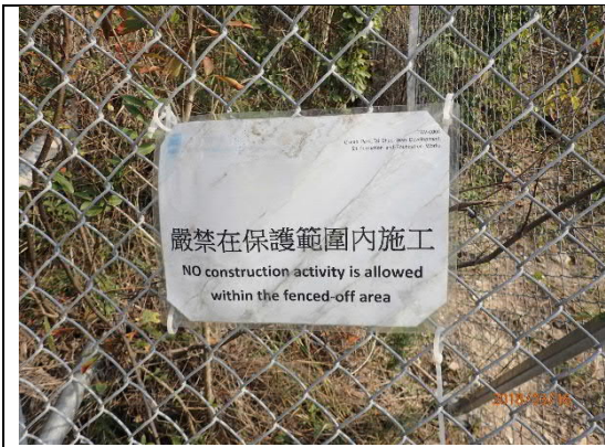
Photo 1 – Current situation of fencing and warning sign
