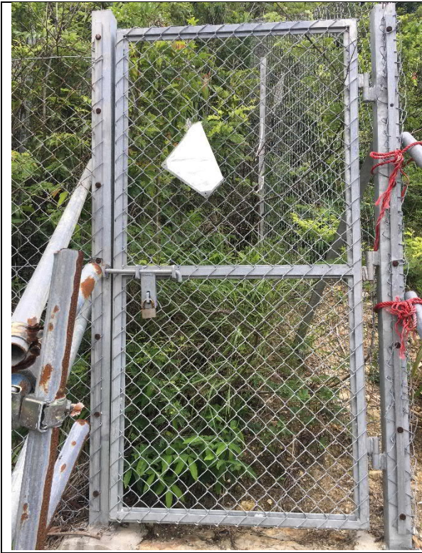
Photo 3 – Current situation of fencing and warning sign
