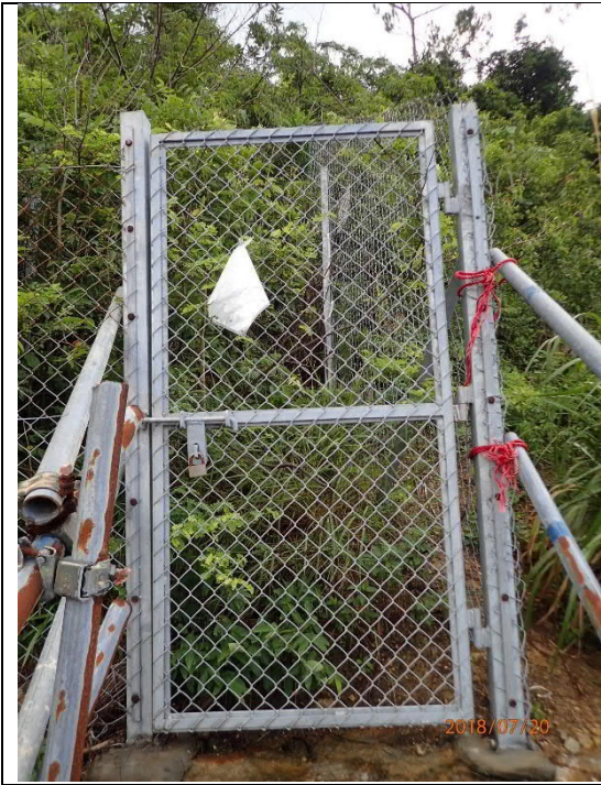
Photo 3 – Current situation of fencing and warning sign
