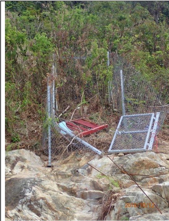
Photo 1 – The preventive mitigation measure was damaged due to super typhoon
