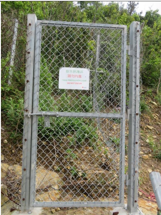
Photo 2 – Current situation of fencing and warning sign
