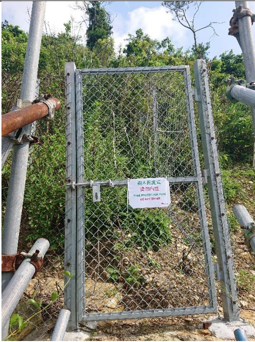
Photo 2 – Current situation of fencing and warning sign
