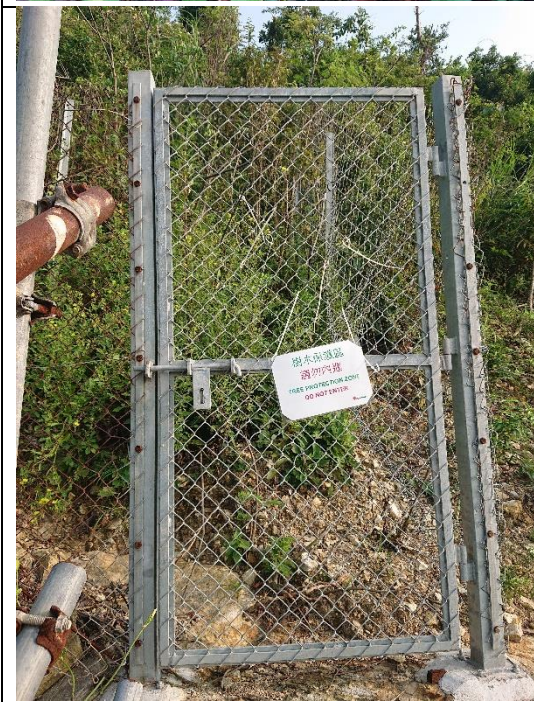
Photo 2 – Current situation of fencing and warning sign
