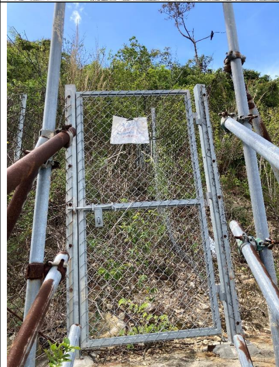
Photo 2 – Current situation of fencing and warning sign
