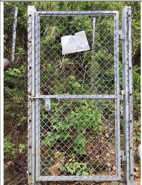
Photo 2 – Current situation of fencing and warning sign
