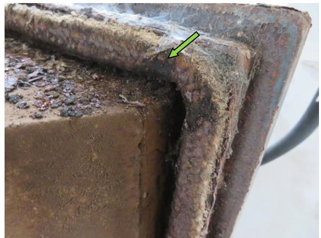
Photo N10. Non-ACM door seal, photo taken at Cage Cleaning Area, 5/F, UPB.
