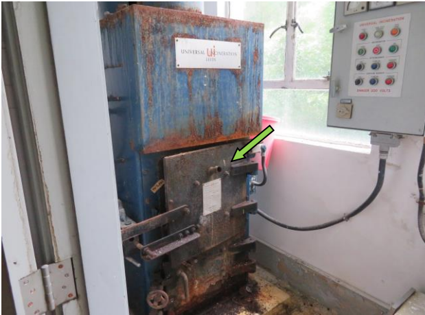
Photo N1. Incinerator, photo taken at Cage Cleaning Area, 5/F, UPB.
