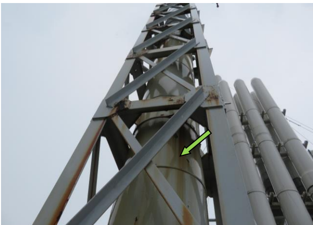
Photo N5. Metal exhaust chimney, photo taken at R/F, UPB.
