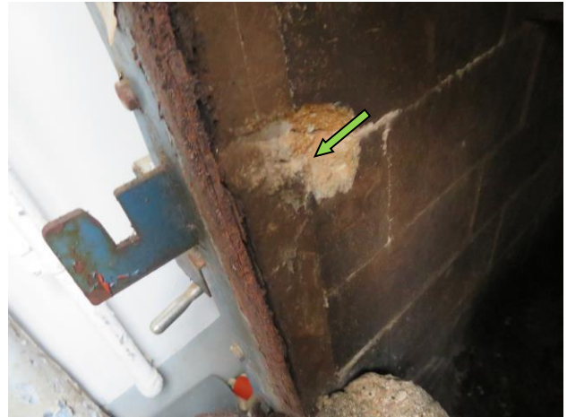
Photo N8. Non-ACM brick inside incinerator, photo taken at Cage Cleaning Area, 5/F, UPB.
