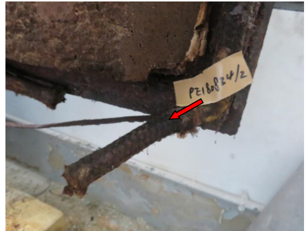
Photo S2. Door seal, (PE180834/2), sampled at Cage Cleaning Area, 5/F, UPB, was confirmed as non-ACM.
