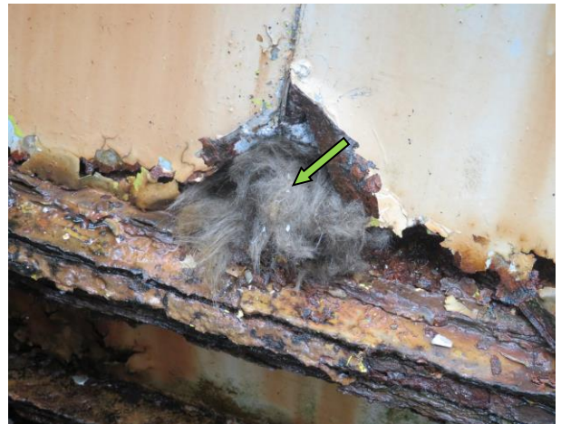
Photo N4. Exhaust Chimney with glass fibre insulation, photo taken at, R/F, UPB.
