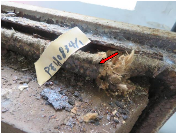
Photo S1. Door seal, (PE180834/1), sampled at Cage Cleaning Area, 5/F, UPB, was confirmed as non-ACM.
