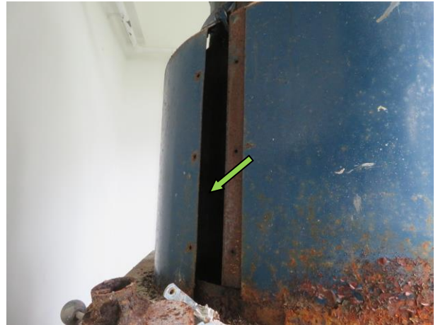
Photo N2. Exhaust Chimney with no insulation, photo taken at Cage Cleaning Area, 5/F, UPB.
