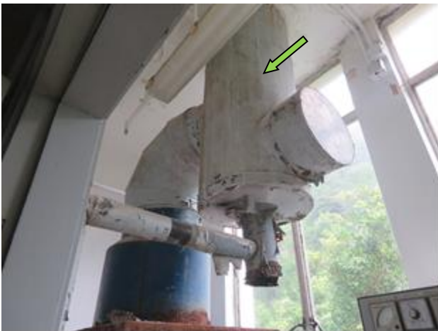
Photo N3. Metal exhaust chimney, photo taken at Cage Cleaning Area, 5/F, UPB.
