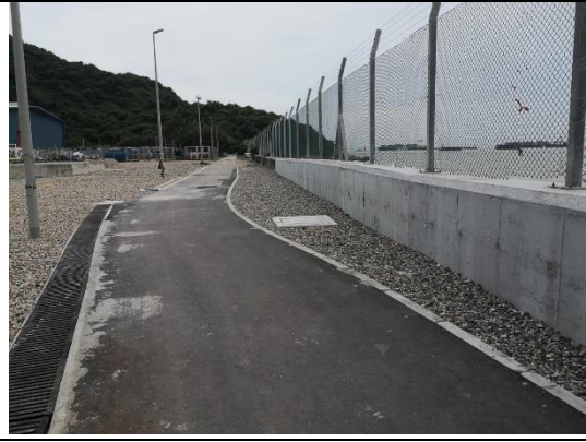
Asphalt pavement has been provided on site to minimize runoff
