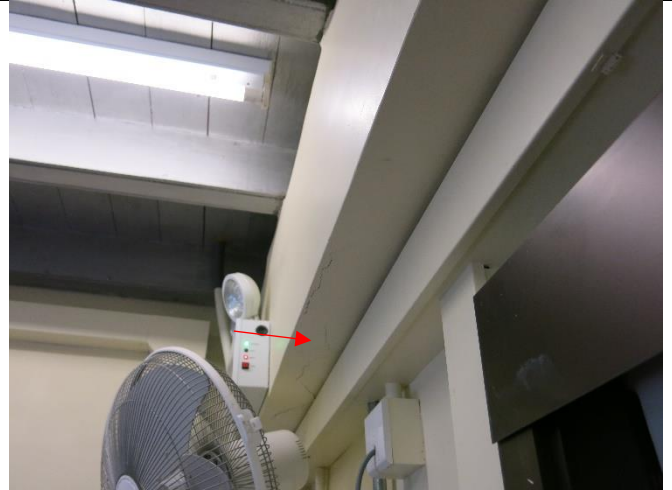
Photo 8: No crack monitoring devices were found at locations as recommended in the approved survey report of NP-11
