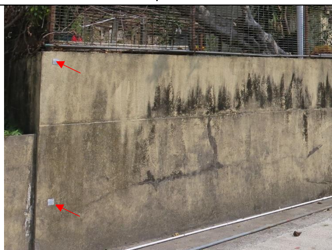
Photo 4: Reflective targets for settlement monitoring were installed on the fence wall at NP-10
