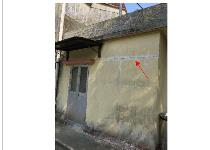
Photo 5: No crack monitoring devices were found at locations as recommended in the approved survey report of NP-10
