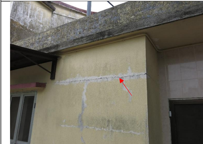
Photo 5: No crack monitoring devices were found at locations as recommended in the approved survey report of NP-10
