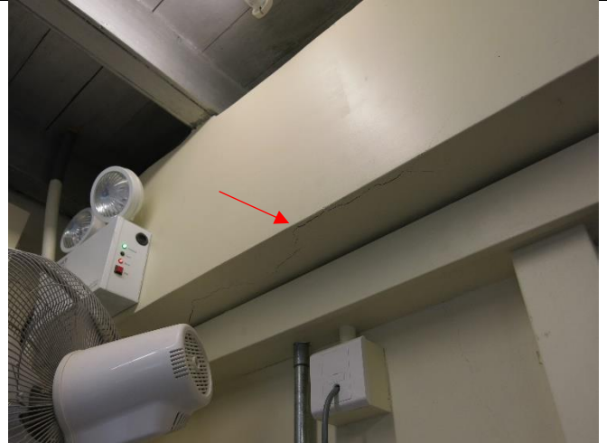
Photo 8: No crack monitoring devices were found at locations as recommended in the approved survey report of NP-11
