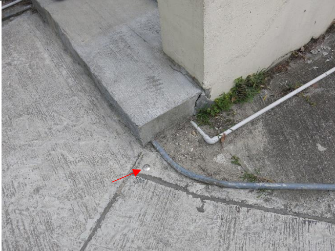
Photo 7: Ground settlement marker for settlement monitoring was installed at the entrance of NP-11
