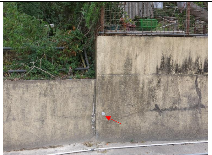
Photo 4: Reflective target for settlement monitoring was installed on the fence wall at NP-10 (missing one reflective target compared to last month)
