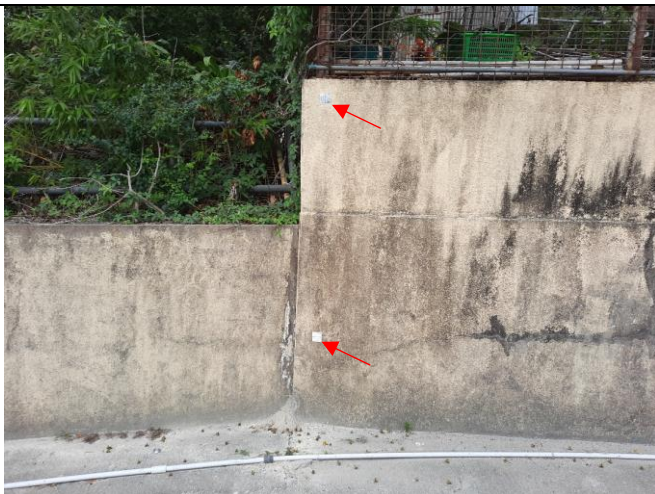
Photo 3: Reflective targets for settlement monitoring were installed on the fence wall at NP-10.
