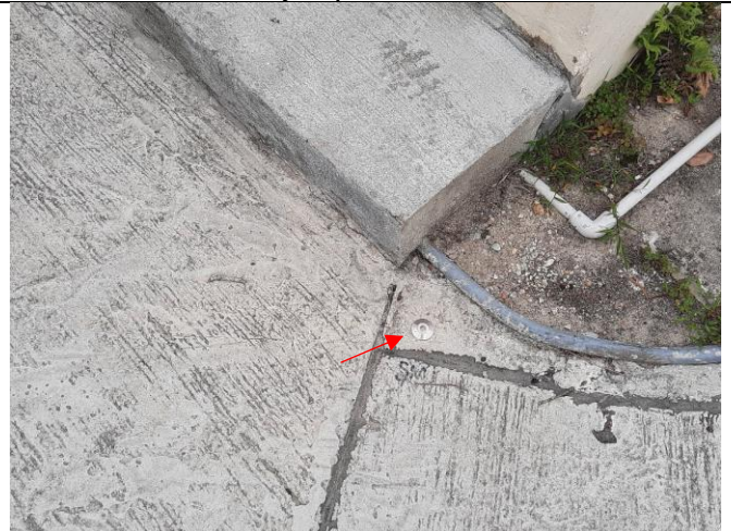
Photo 6: Ground settlement marker for settlement monitoring was installed at the entrance of NP-11.
