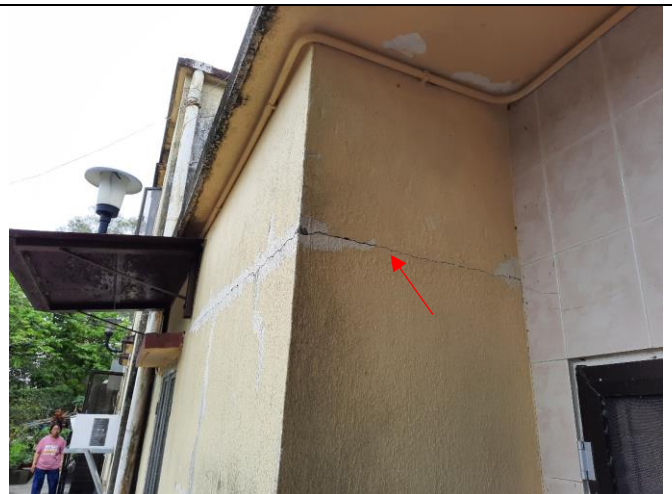
Photo 4: No crack monitoring devices were found at locations as recommended in the approved survey report of NP-10.
