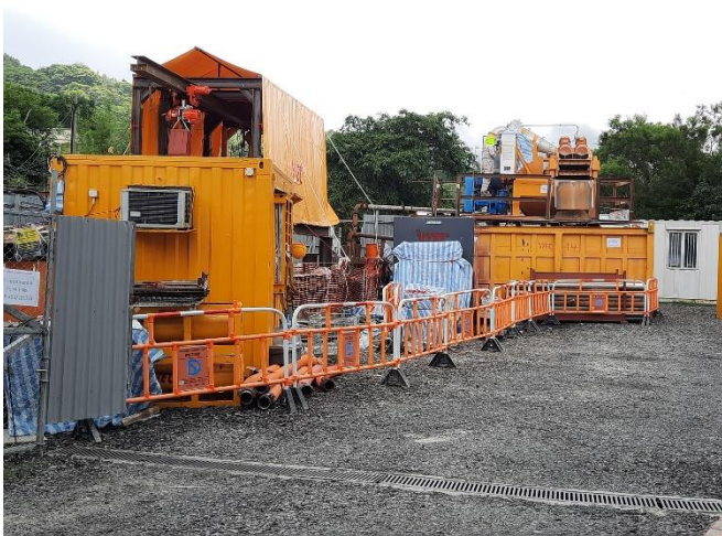
Photo 1: The jacking pit in the opposite of NP-10 has been constructed. Works in progress.
