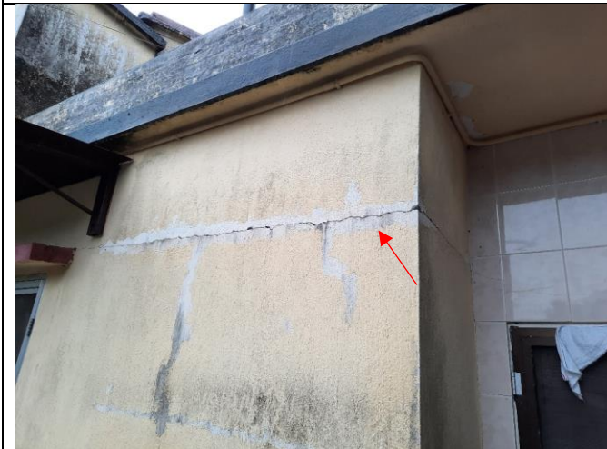
Photo 4: No crack monitoring devices were found at locations as recommended in the approved survey report of NP-10.
