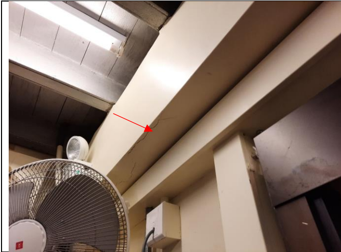
Photo 7: No crack monitoring devices were found at locations as recommended in the approved survey report of NP-11.
