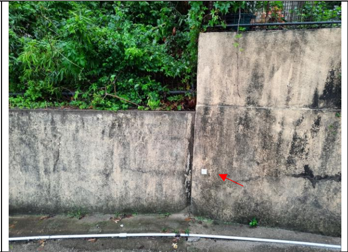
Photo 3: Reflective target for settlement monitoring was installed on the fence wall at NP-10 (missing one reflective target compared to last month)
