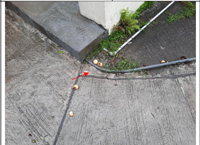
Photo 6: Ground settlement marker for settlement monitoring was installed at the entrance of NP-11.
