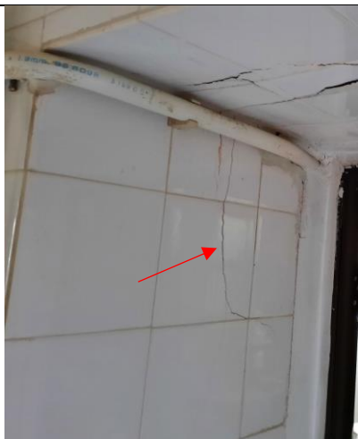
Photo 4: NP-10 (D64): Location for installation of tell-tale (1no.) agreed by ET and Contractor during site audit.
