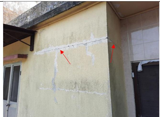
Photo 3: NP-10 (D18): Locations for installation of tell-tales (2nos.: 1no. on each side of the wall) agreed by ET and Contractor during site audit.
