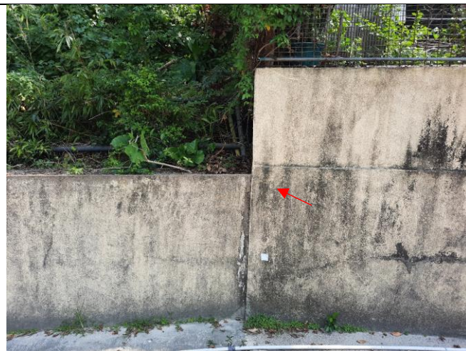
Photo 2: Reflective target for settlement monitoring was installed on the fence wall at NP-10 (missing one reflective target compared to May 2021).
