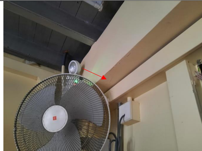
Photo 8: NP-11: Location for installation of tell-tale (1no.) agreed by ET and Contractor during site audit.
