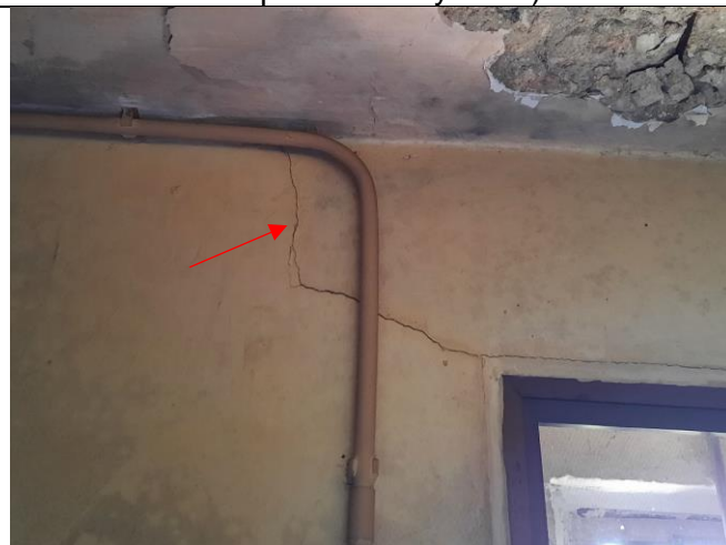
Photo 5: NP-10 (D92): Location for installation of tell-tale (1no.) agreed by ET and Contractor during site audit.
