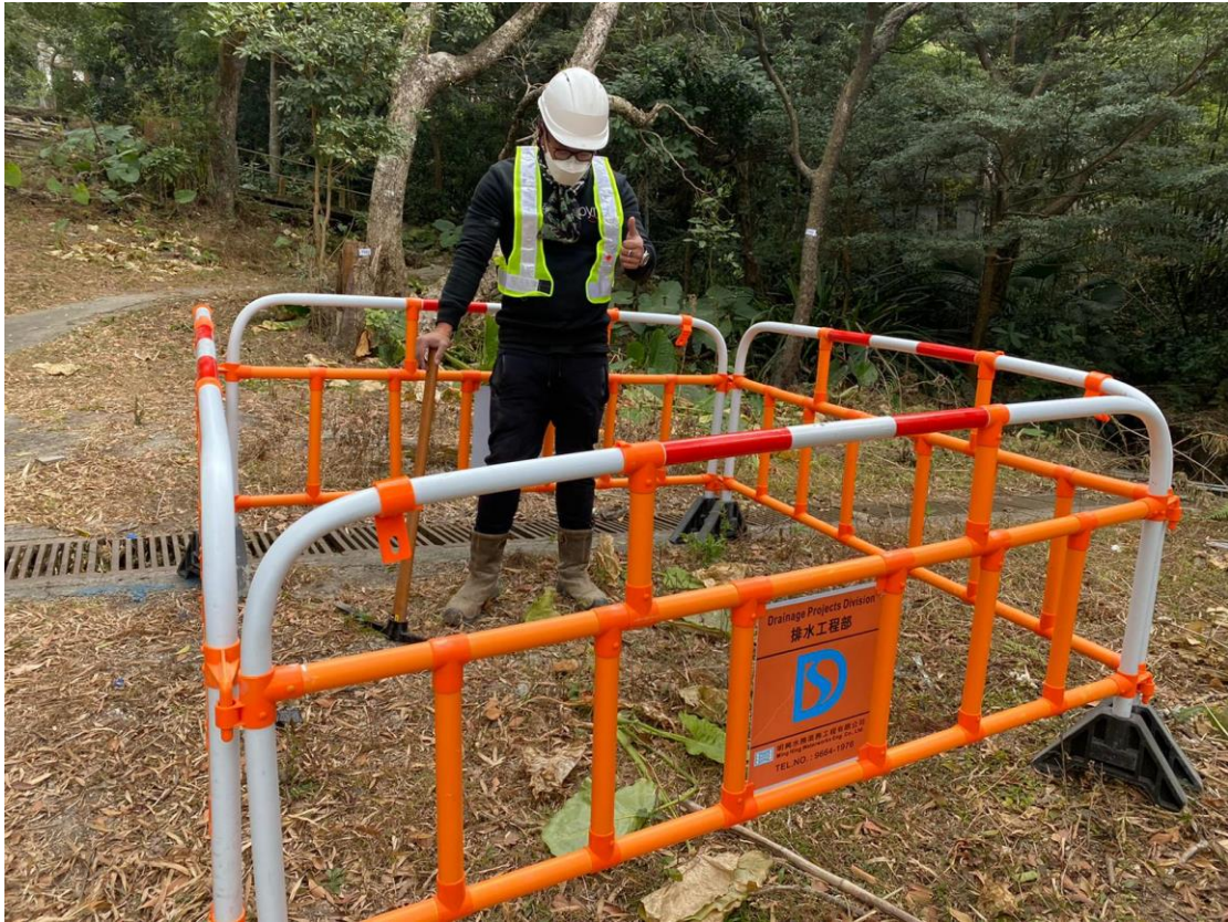
Appendix E1: Construction barriers that shall be erected for the No-intrusion Zone.
