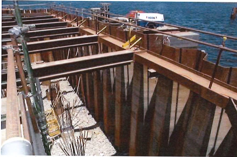
Completely dry excavation was able to be carried out due to grouted clutches
