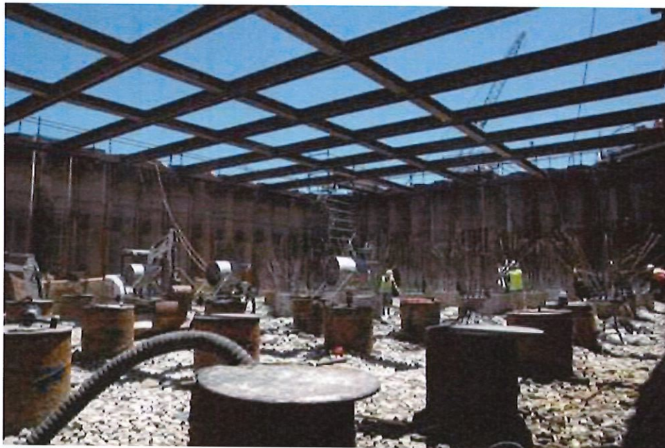
The plastic sealant application allowed the construction to be carried out unobstructed and in the dry condition
