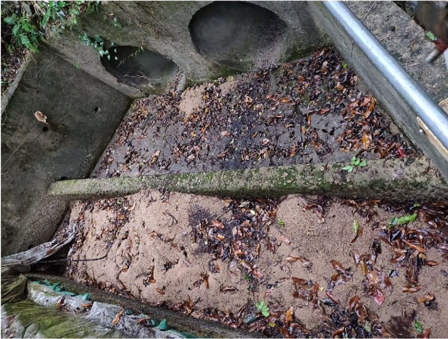
Photograph taken on 2 February 2022 at monitoring location C2. Running water from upstream is allowed via cement drainage pipe.
