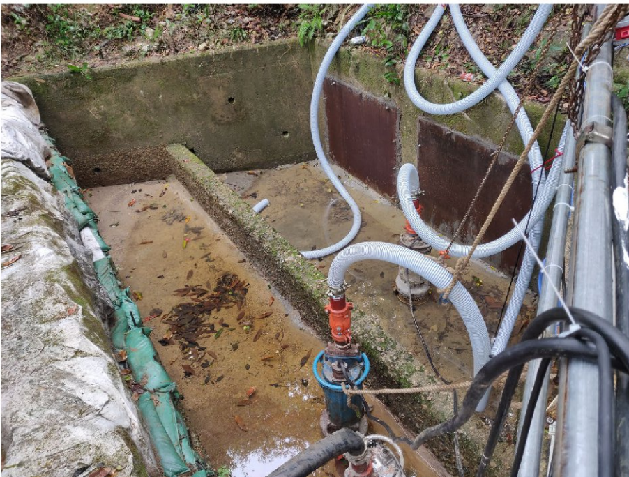
Photograph taken on 7 March 2022 at monitoring location C2. Water is accumulated because of the blockage of cement drainage pipe.
