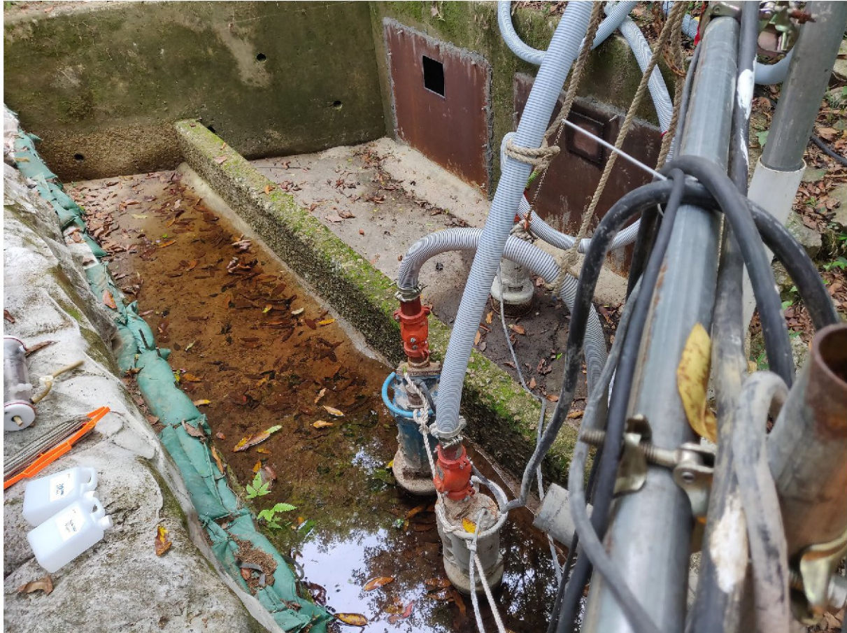
Photograph taken on 7 May 2022 at monitoring location C2. Water is accumulated because of the blockage of cement drainage pipe.
