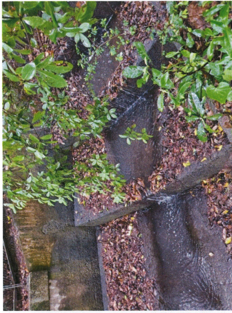
2021.06.22_C1b & C1b# Not Enough Water
